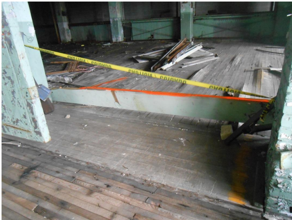
Photo No. 4 – South Building: Barricade Tape and Plywood Restricting Access
