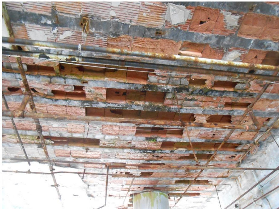
Photo No. 16 – North Building: Deteriorated Hollow Clay Roof Tile
