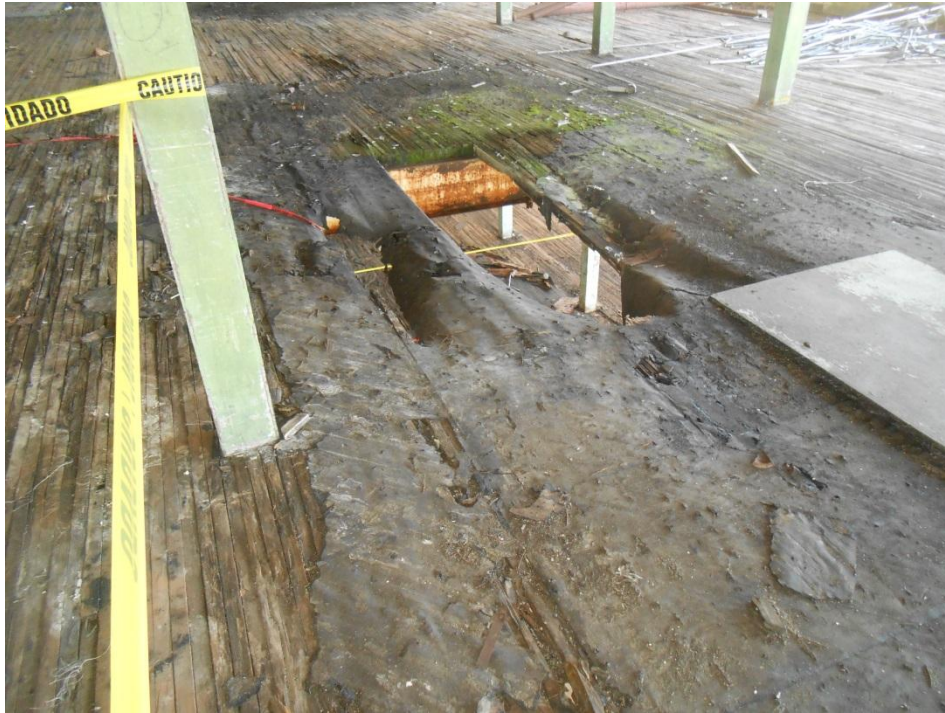
Photo No. 7 – South Building: Timber Decking Collapse at 5 th Floor
