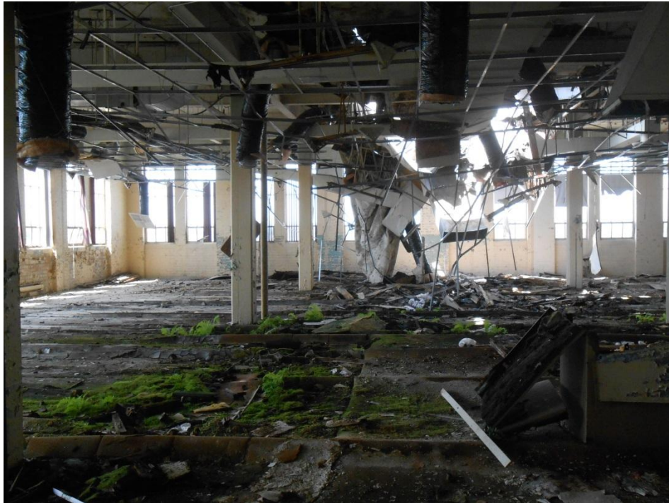
Photo No. 9 – South Building: Roof Deck Collapse in Southwest Corner
