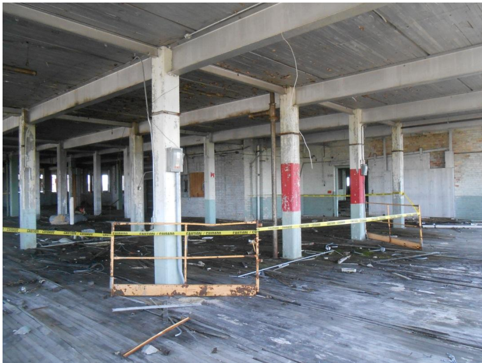
Photo No. 8 – South Building: Restricted Area at 6 th Floor Collapse
