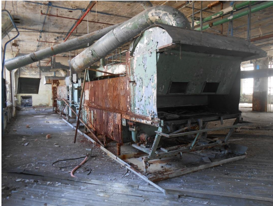
Photo No. 13 – North Building: Existing HVAC Equipment
