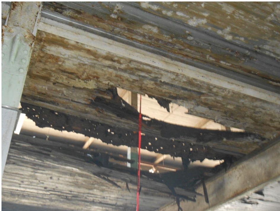
Photo No. 6 – South Building: Timber Decking Collapse at 4 th Floor
