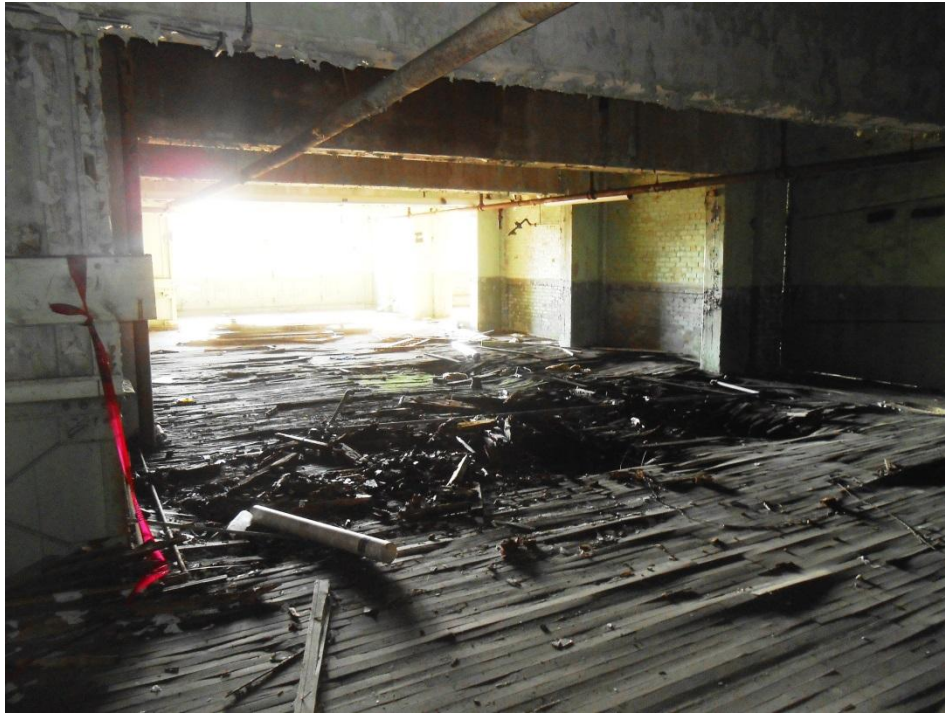
Photo No. 3 – South Building: 2 nd Floor Timber Decking Collapse
