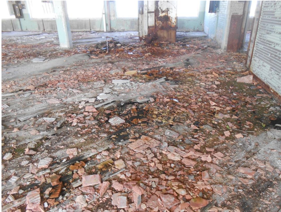
Photo No. 15 – North Building: Hollow Clay Roof Tile Debris on 6 th Floor
