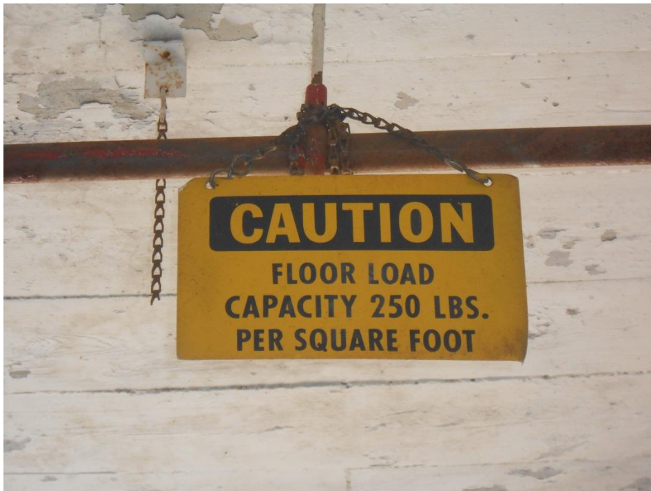
Photo No. 14 – North Building: Maximum Floor Live Load Posting
