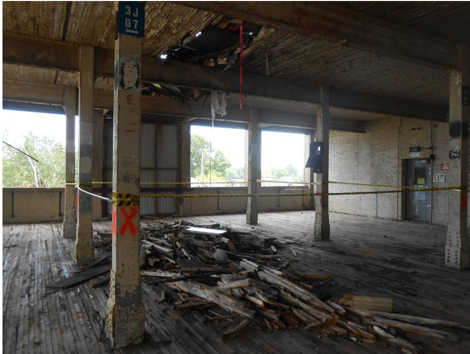
Photo No. 5 – South Building: Timber Decking Collapse at 3 rd Floor
