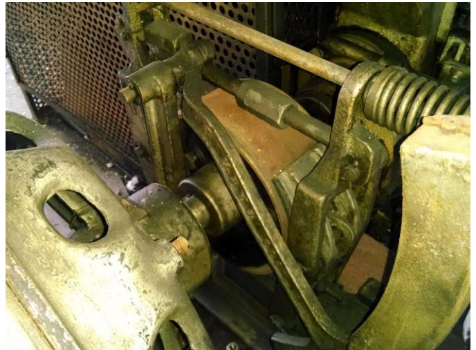
Photo 29: Elevator Brake Shoe (representative)
