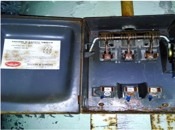
Photo 7: Square D – Transite Panel
