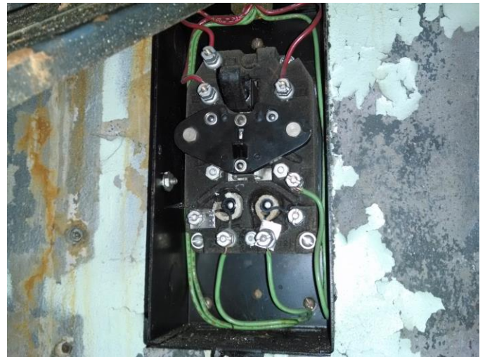
Photo 11: Cutler Hammer – Motor Control
