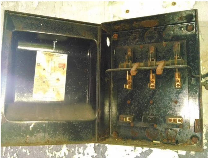
Photo 14: Square D: Small Black Isolators
