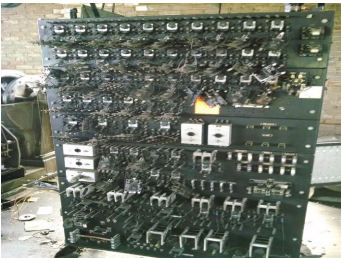
Photo 27: Elevator Electrical (representative)
