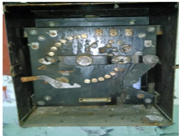
Photo 12: GE Slate Electrical Panel
