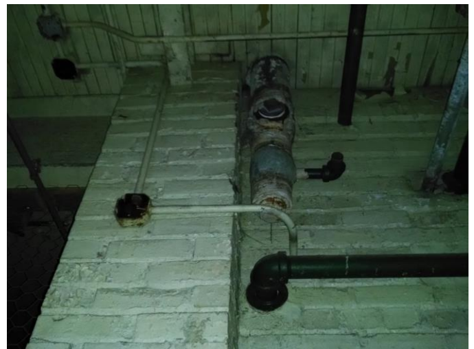
Photo 24: Pipe Insulation & Pipe Fittings (representative)
