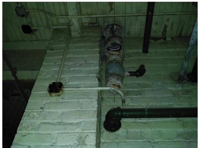
Photo 24: Pipe Insulation & Pipe Fittings (representative)
