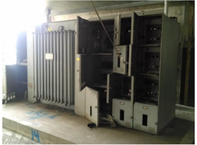
Photo 16: Large Transformer: Black Box Electrical
