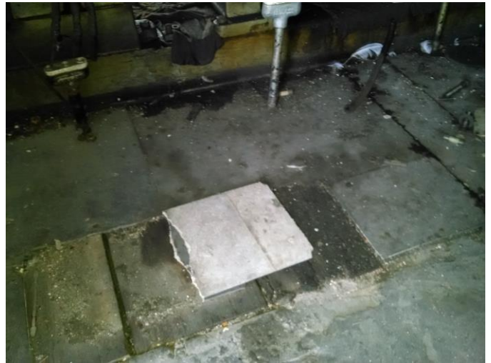
Photo 28: Elevator Transite (representative)
