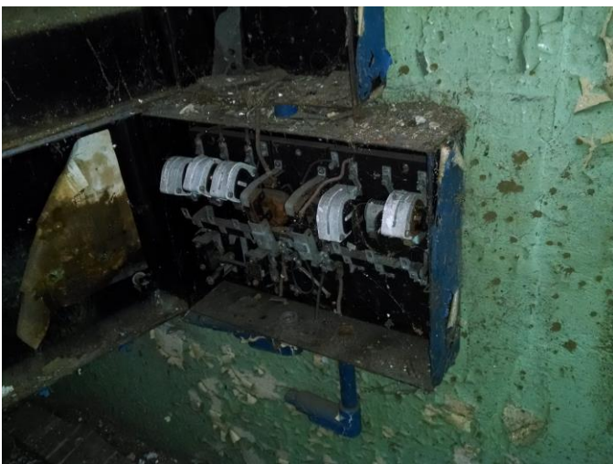
Photo 15: Cutler Hammer: White Isolator
