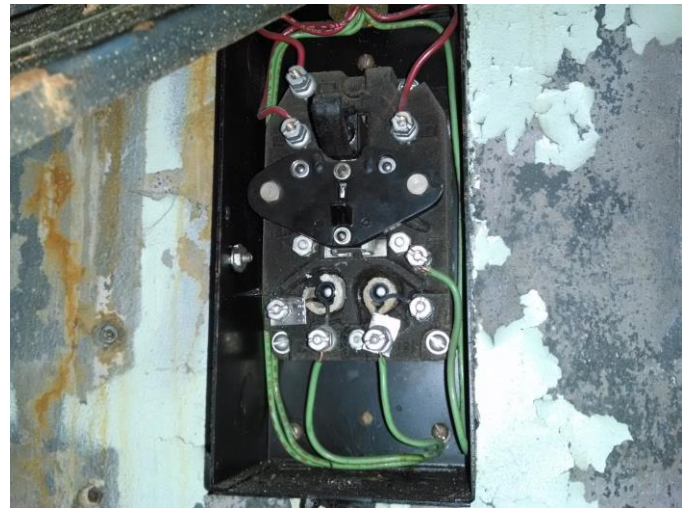
Photo 11: Cutler Hammer – Motor Control
