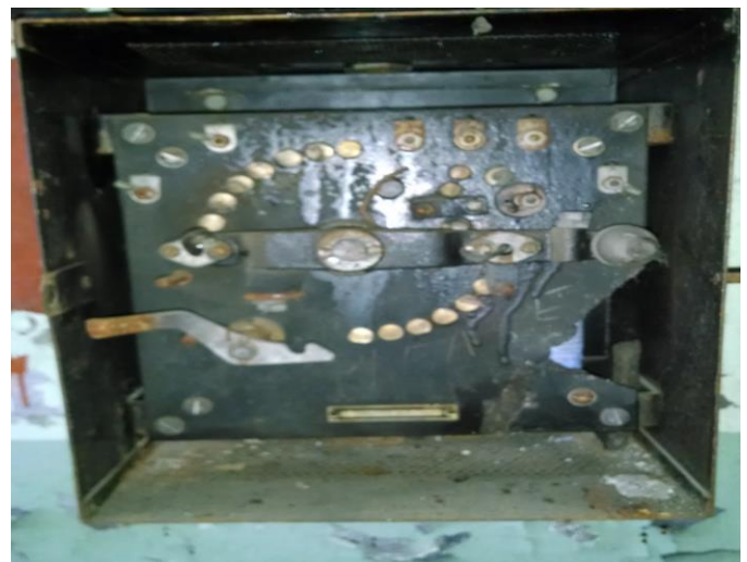
Photo 12: GE Slate Electrical Panel
