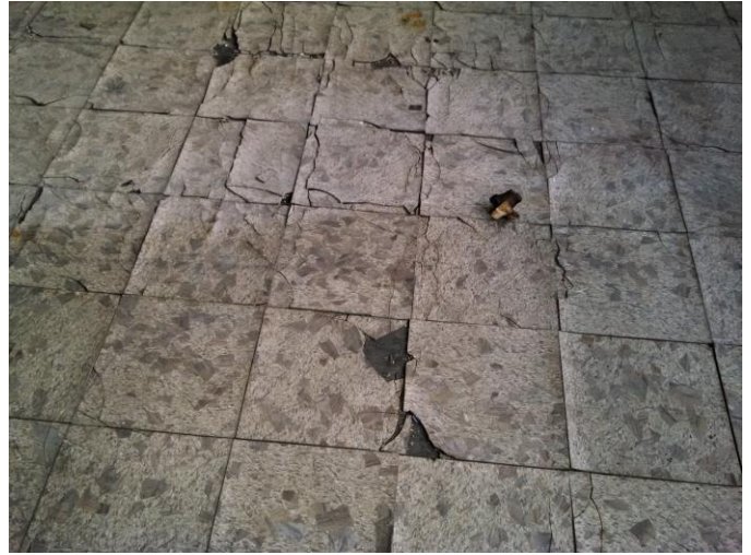
Photo 22: 12" Tan Floor Tile
