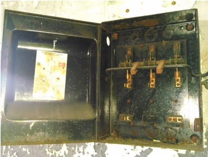
Photo 14: Square D: Small Black Isolators
