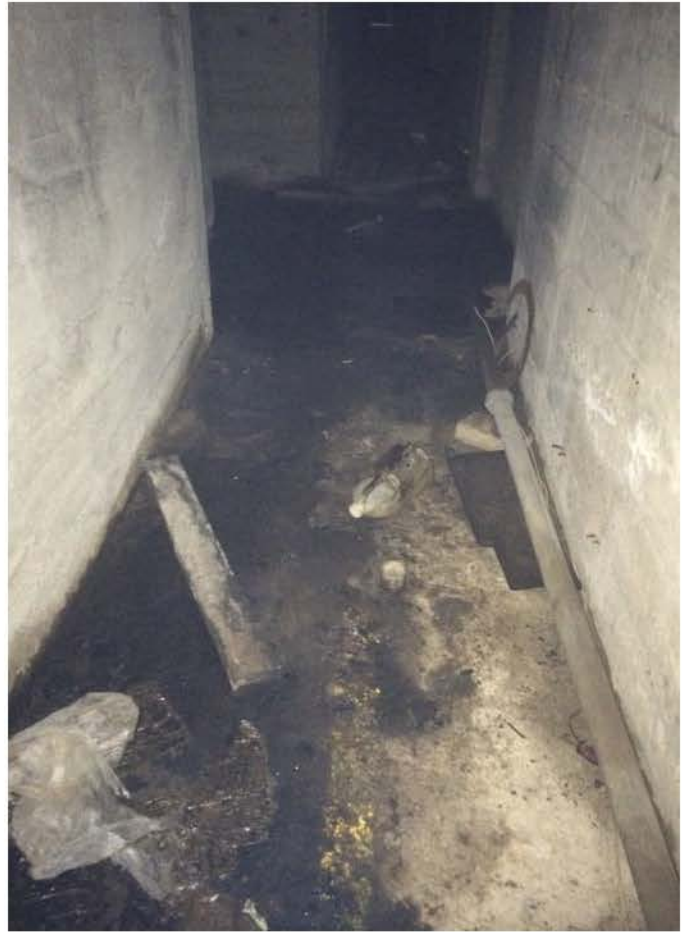
#6 - Debris and sludge in tunnel by heat treating pit
