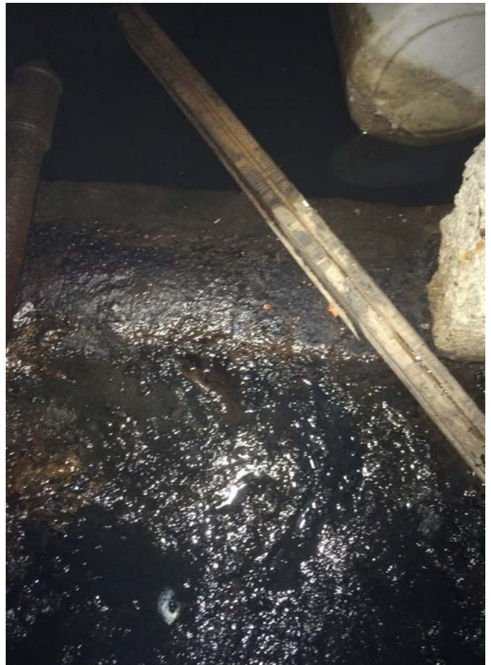
#4 - Sludge in doorway from tunnel to heat treating pit
