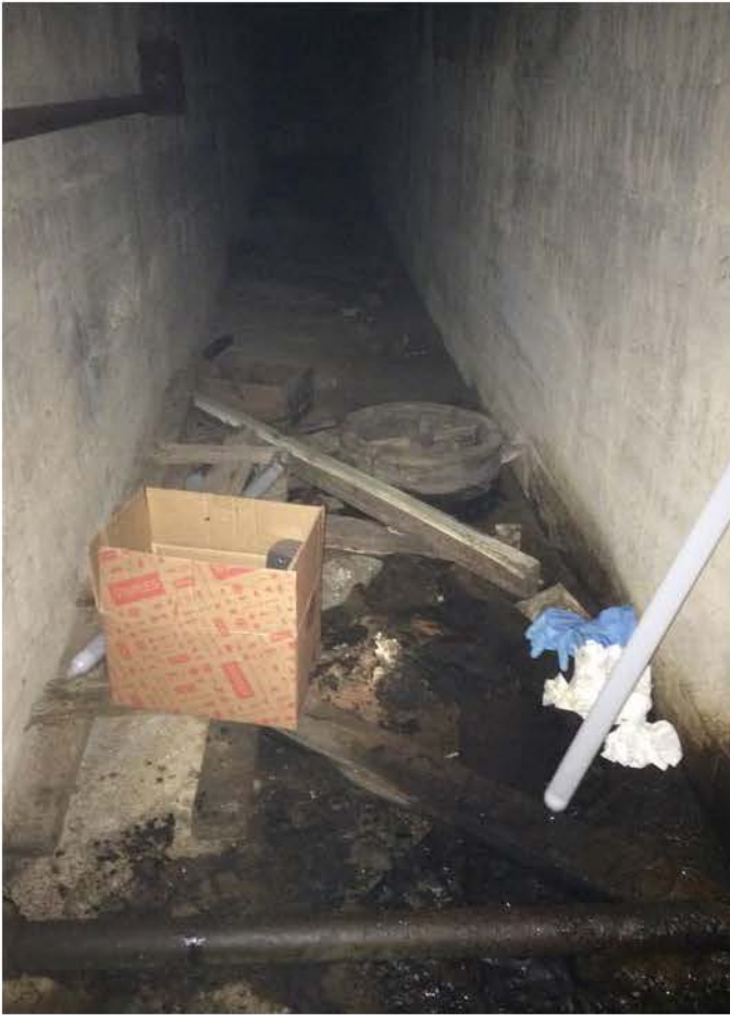
#5 - Debris and sludge in tunnel by heat treating pit
