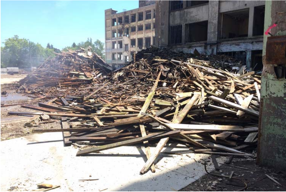
#3 - Debris pile by Loading Dock prior to removal
