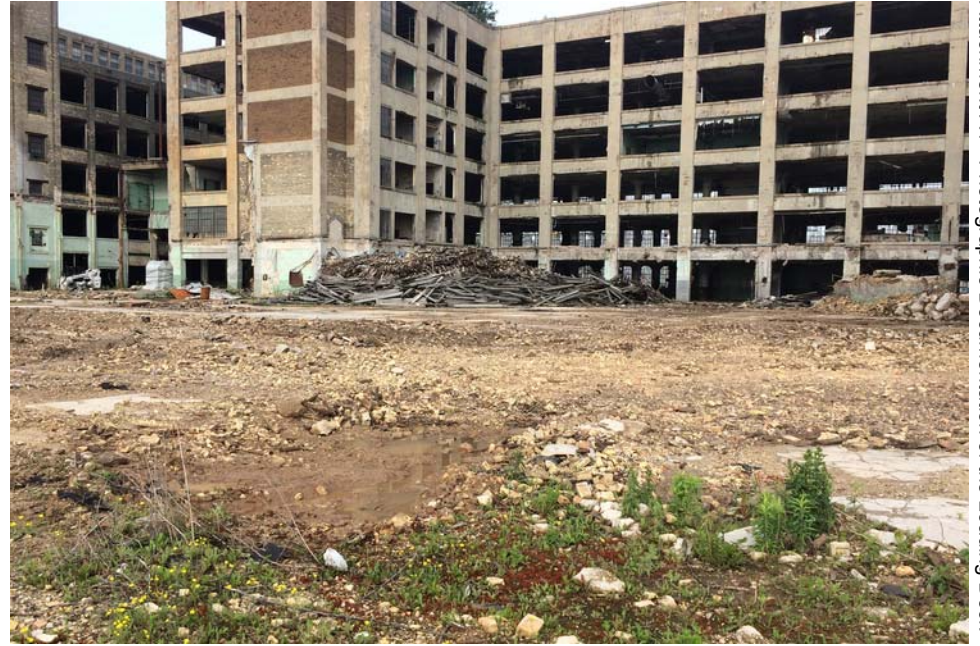
#1 - Debris pile by Loading Dock prior to removal
