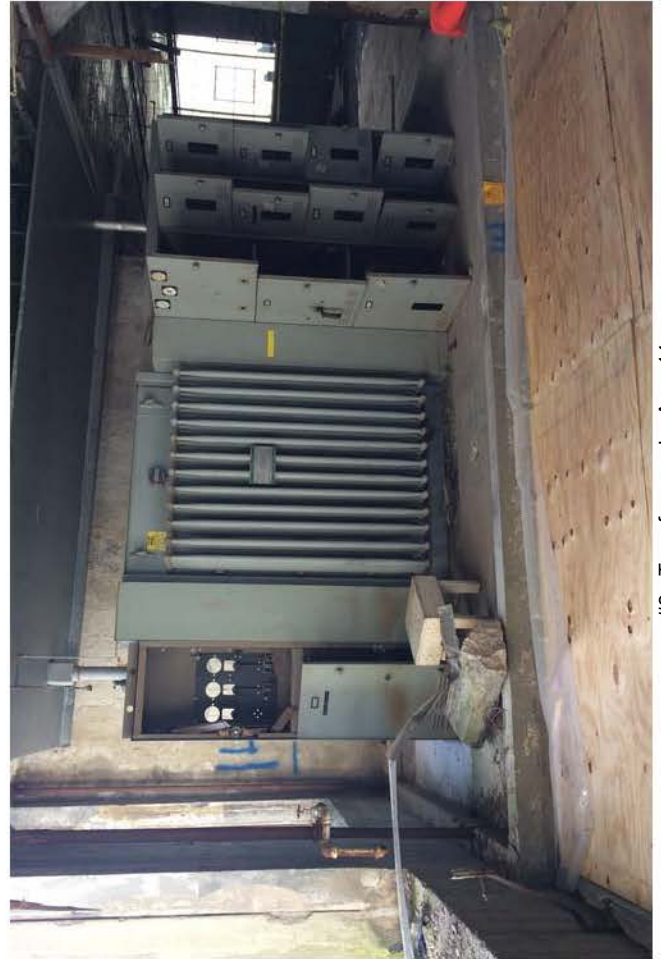
#2 - Transformer by Area 14
