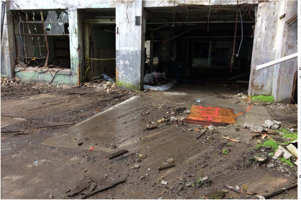
#5 - Former debris pile by the Loading Dock
