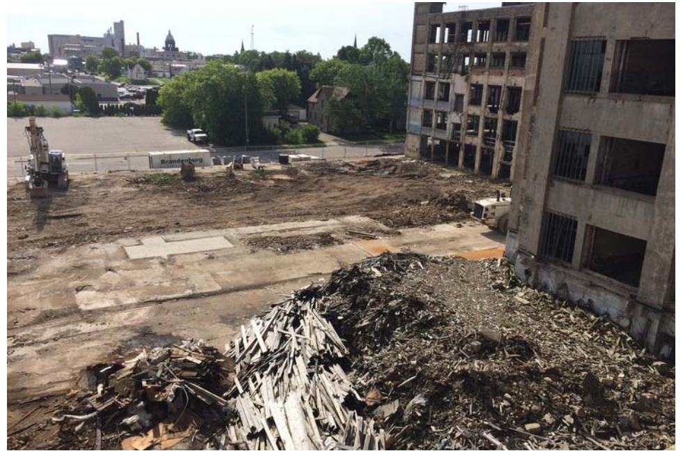
#2 - Debris pile prior to removal
