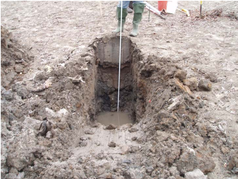
Photo #14. Test Pit #2, note surface water infiltration approximately 4 feet from the surface.
