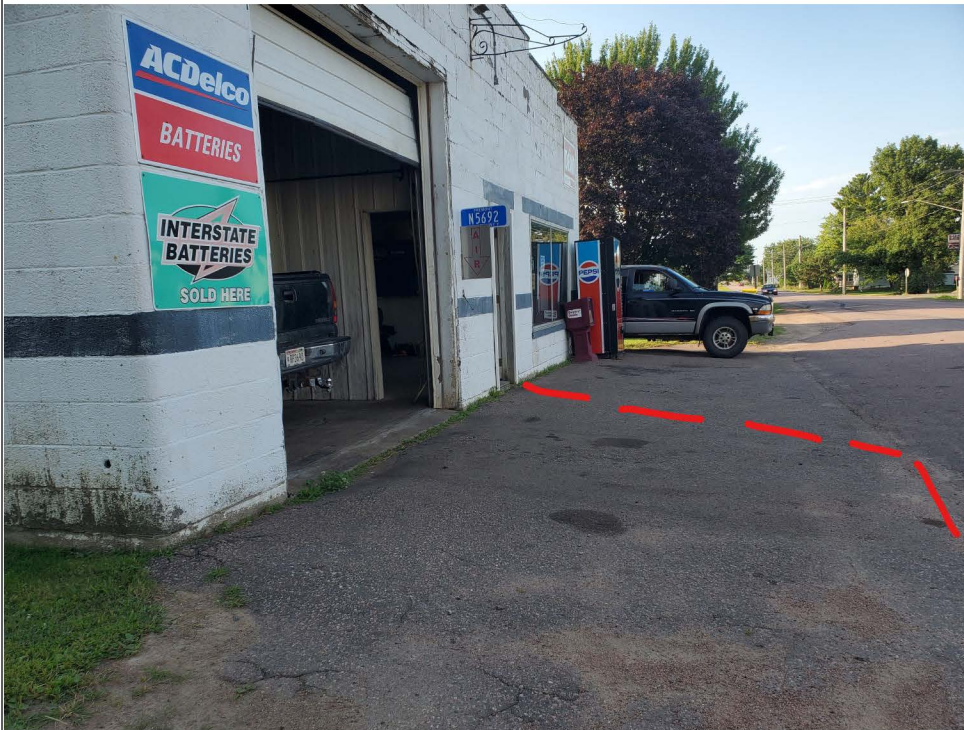
Title: Chili Service & Strey Property, 03-10-545214, 08/21/2020. Photo taken from northwestern corner of property. View is facing south. Minor cracks in cap. Cap extent confined by dashed red line (approx.). Building still in place.
