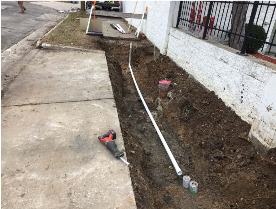
Photo 1: 2-inch PVC piping from MW21/SVE2 toward SVE blower Photo Direction: South Date: 3/16/2020
