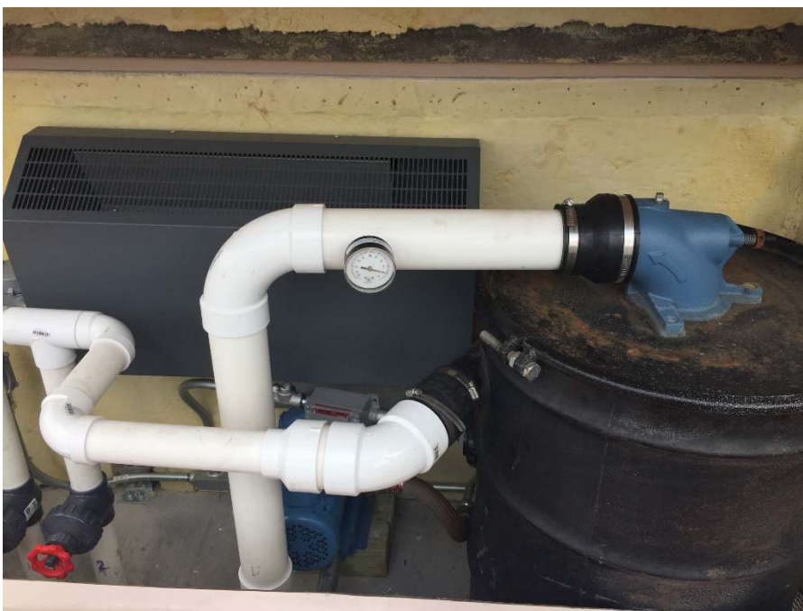
Photo 6: Interior piping of SVE enclosure. Note piping from SVE wells on left, Knockout tank on right, SVE blower at the bottom. Photo Direction: East Date: 4/9/2020
