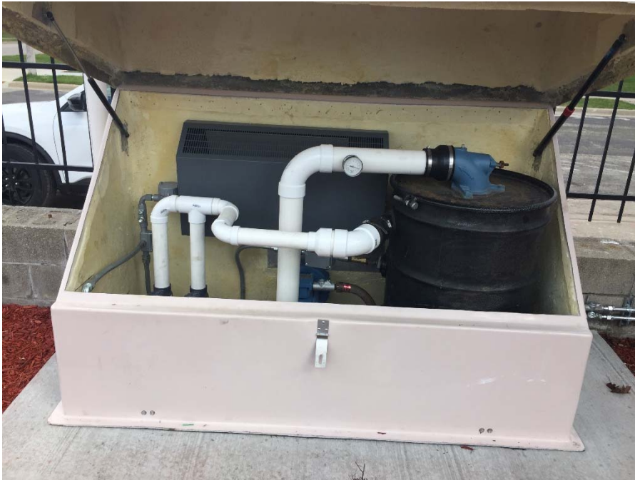
Photo 5: Interior piping of SVE enclosure. Note knockout tank on right, SVE blower at bottom and explosion-proof heater at back. Photo Direction: East Date: 4/9/2020
