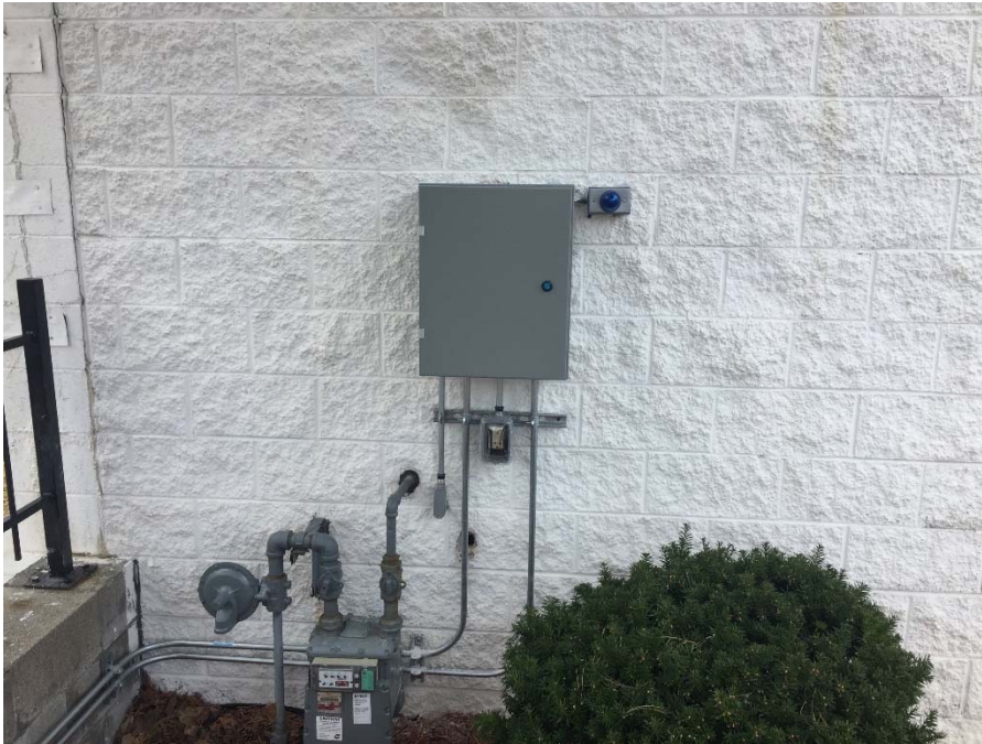
Photo 7: Control Panel mounted on wall of carwash building. Photo Direction: South Date: 4/9/2020
