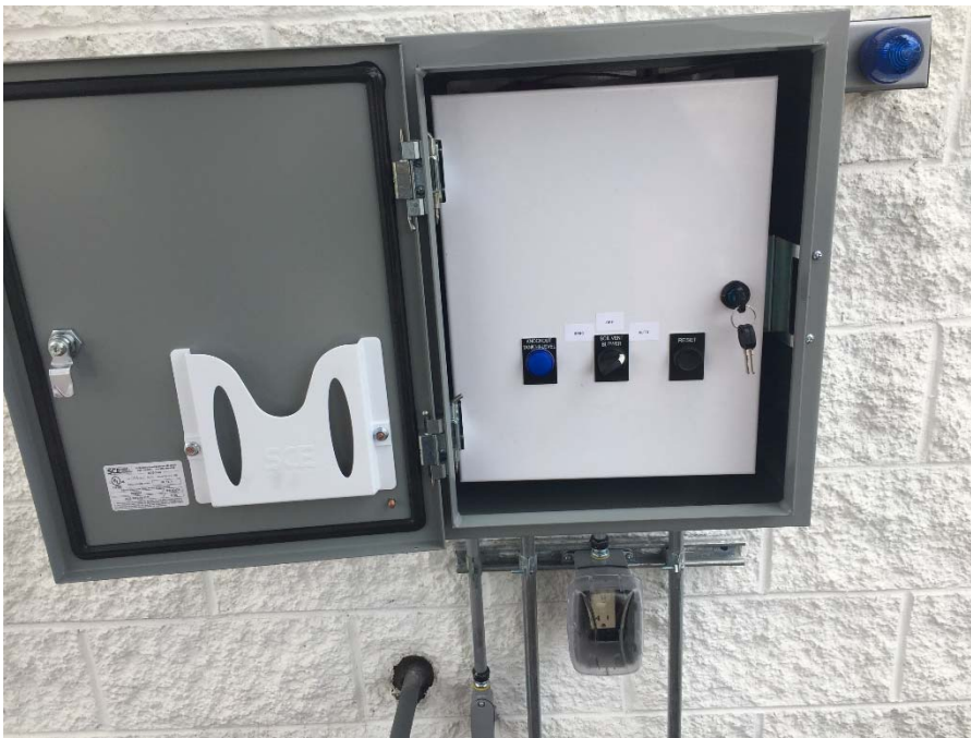
Photo 8: Interior of Control Panel. Photo Direction: South Date: 4/9/2020
