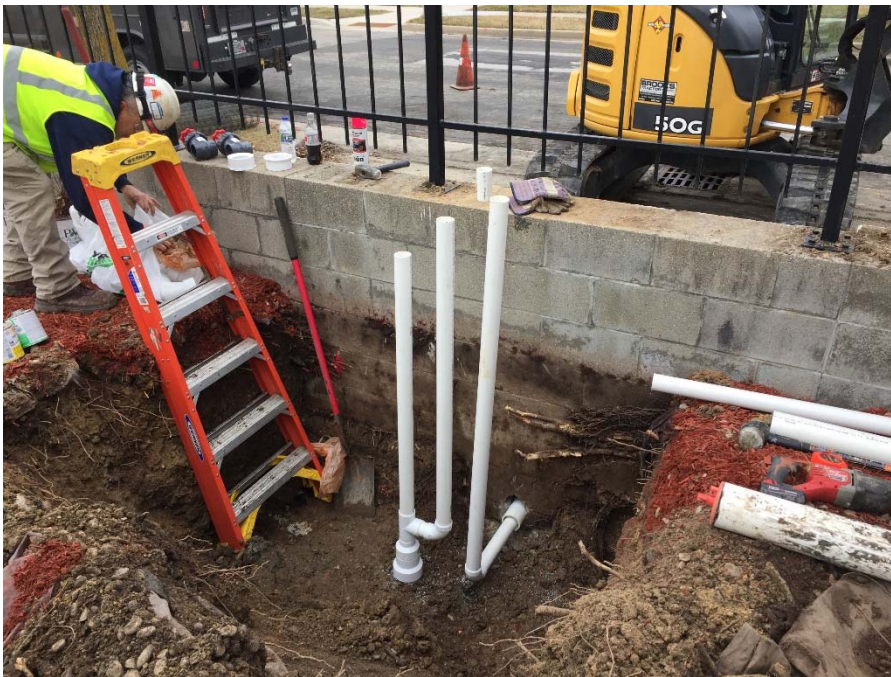
Photo 2: Piping at location of SVE enclosure. Note pipe from MW21/SVE2 coming through wall of retaining wall. Photo Direction: East Date: 3/16/2020
