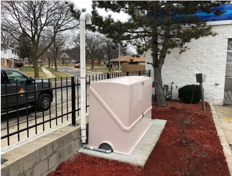
Photo 9: Exterior of SVE enclosure with PVC exhaust piping. Photo Direction: South Date: 4/9/2020
