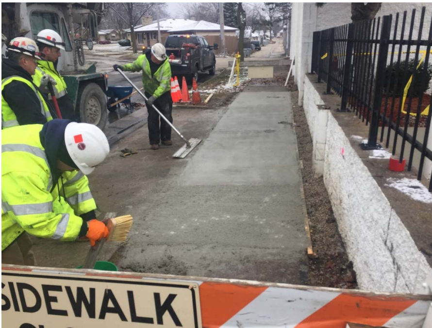
Photo 4: Installing new concrete sidewalk along W. Sarasota Place. Photo Direction: South Date: 3/23/2020
