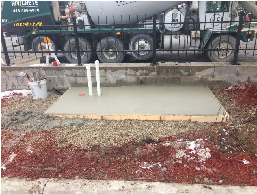
Photo 3: SVE enclosure concrete pad with SVE piping. Photo Direction: East Date: 3/23/2020
