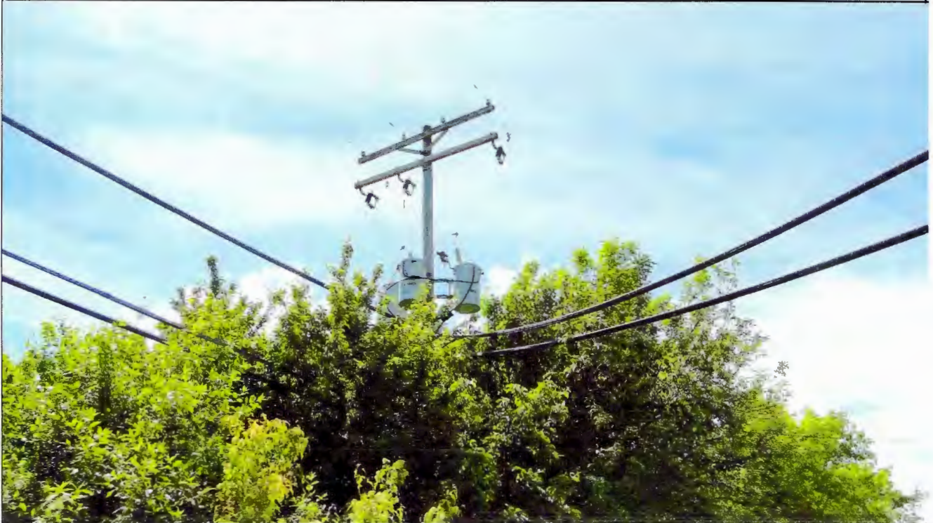
Photo 9: Three pole-mounted transformers between North Main and North Bay Drive properties.
