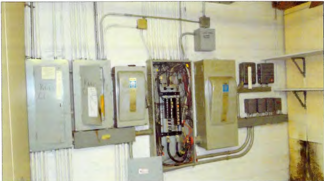
Photo 20: Electrical panels in Unit 2.
