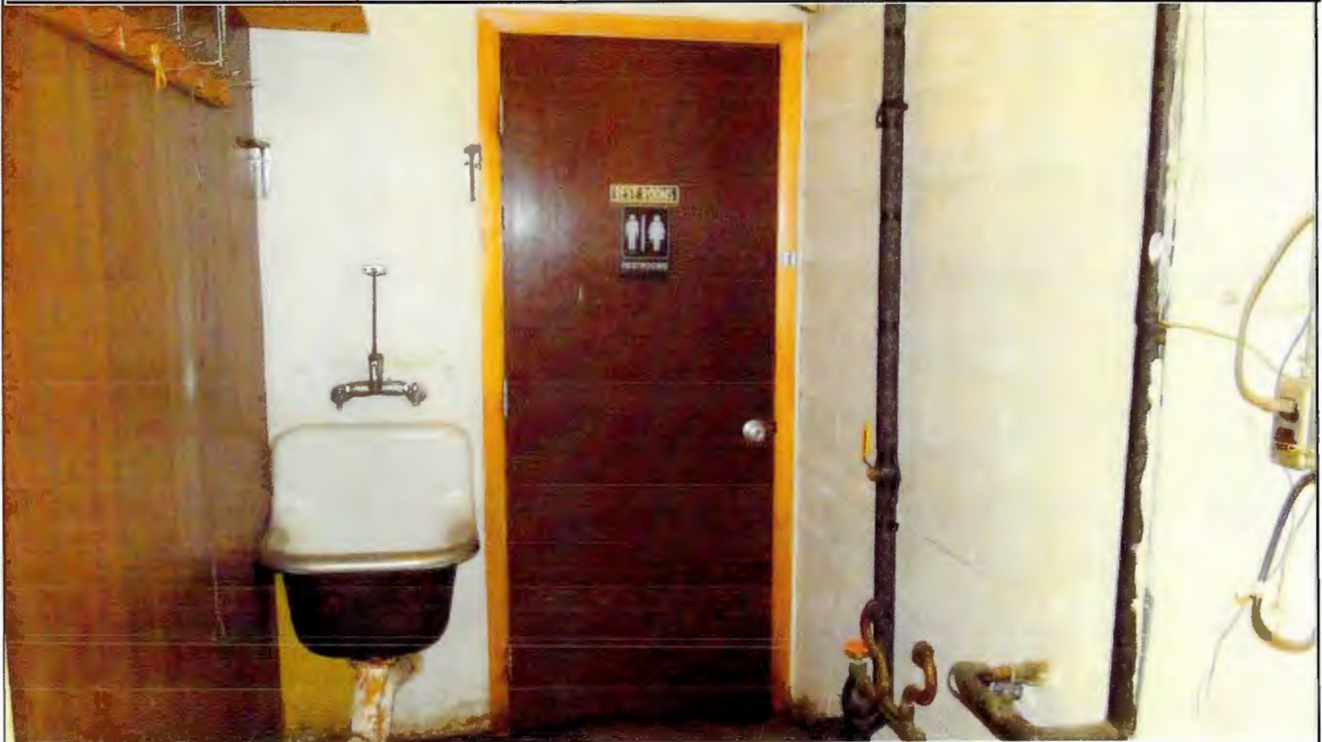
Photo 21: Wash basin in Unit 2.
