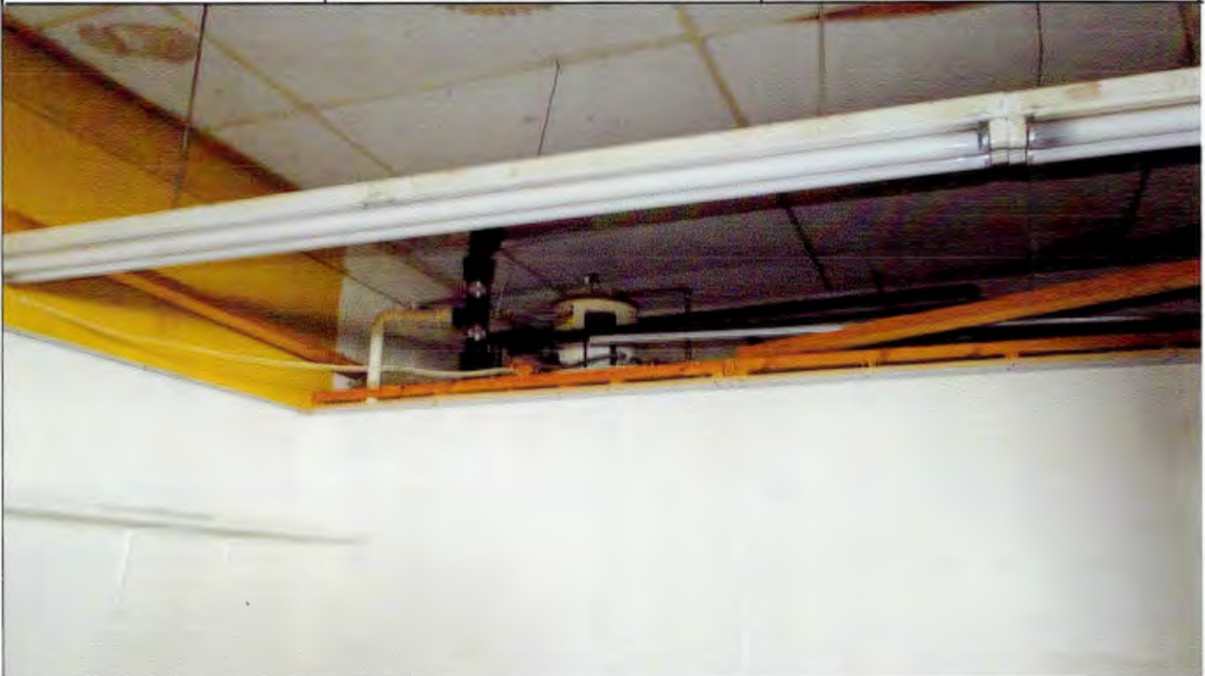
Photo 23: One of two water heaters in Unit 2.
