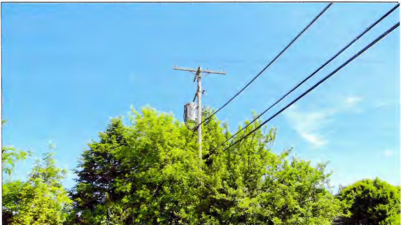
Photo 10: Pole-mounted transformer at northeast corner of North Main Street property.
