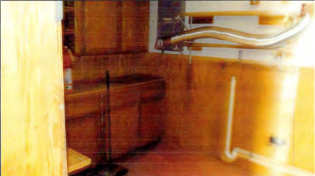
Photo 25: Storage area in Unit 3.
