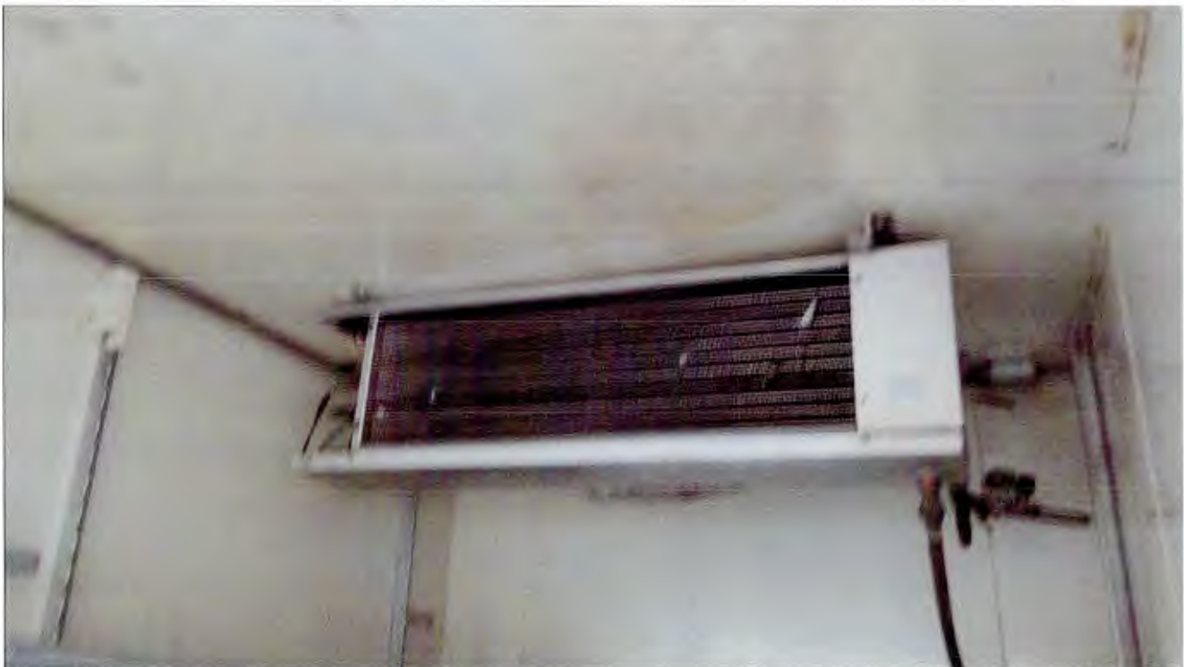
Photo 12: Cooling unit in back room of former convenience store (Unit 2).
