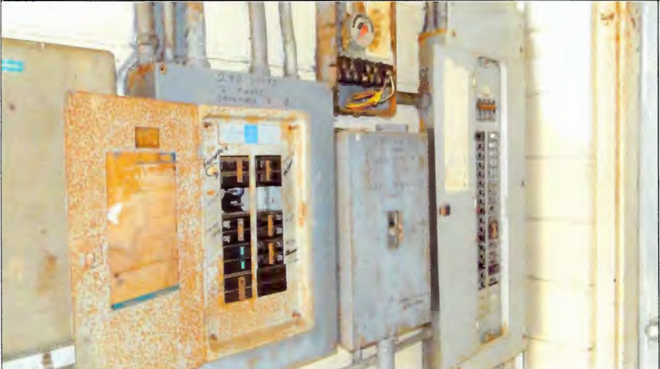
Photo 17: Electrical panels in Unit 1.
