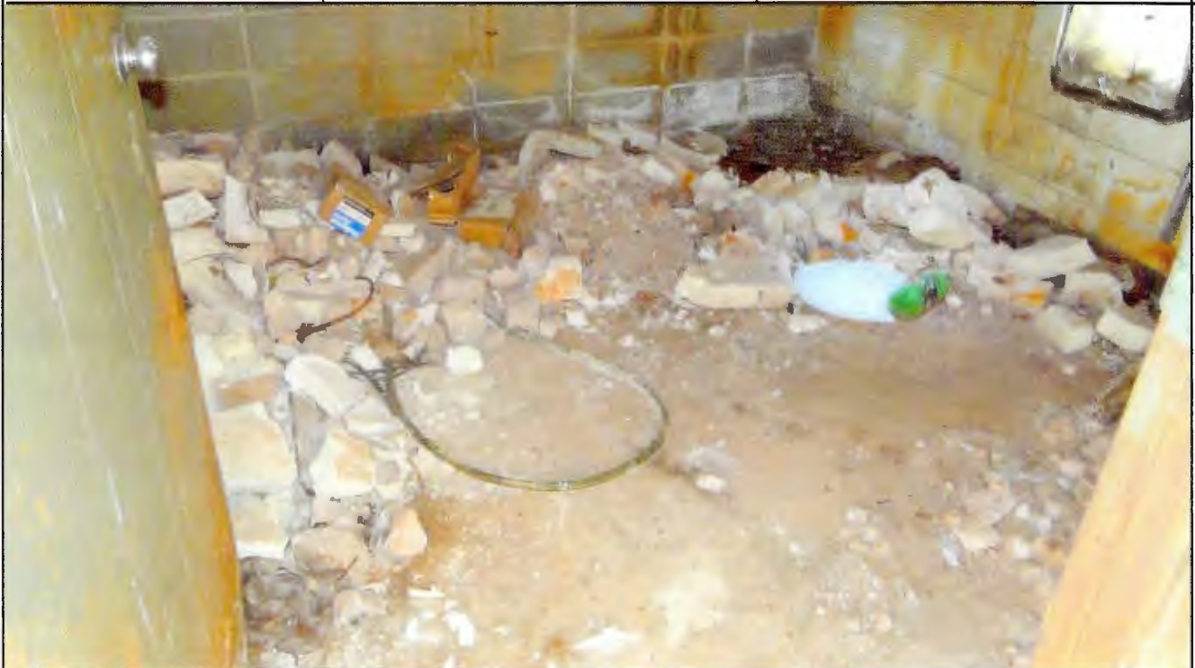
Photo 15: Debris in concrete block room in Unit 1.
