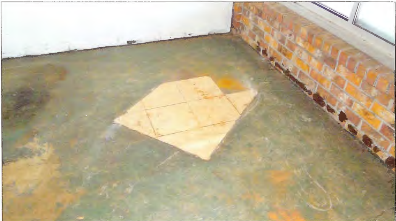
Photo 16: Patch of floor tile left in Unit 1.
