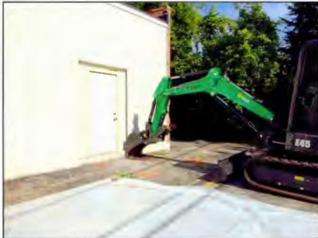
Photo 7. The top asphalt layer was removed by backhoe to expose the contaminated soils below. [Photo taken looking northwest]
