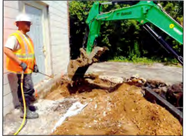
Photo 18. Excavated soils from the upper 2.5 feet were placed back into the excavation and blended with the treatment solution in the same manner as the in-situ soil. The size of the final treatment area was six feet wide (west to east) by five feet long (north to south) by 5 feet deep. [Photo taken looking north]
