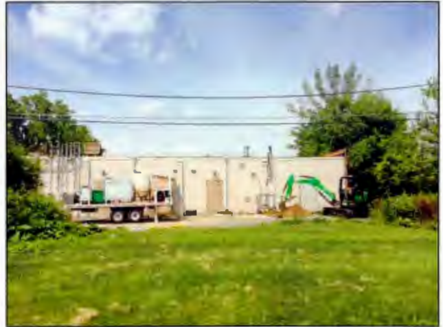
Photo 14. Full view of the pilot test set-up, and the pump truck located south of the treatment area. The pilot test was located immediately outside the back door of the former drycleaning facility at the north end of the building. [Photo taken looking west]
