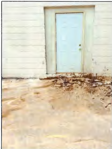
Photo 19. All soils were returned to the excavation and the asphalt placed on top. [Photo taken looking west]
