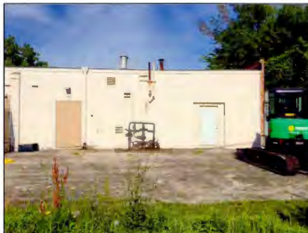
Photo 2. The pilot test location was located immediately outside the back door at the northeast corner of the former dry cleaning establishment.
