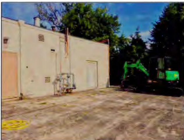
Photo 1. A view of the site prior to pilot test activities. The excavation was moved north several feet from the proposed location to accommodate the outside piping and monitoring well.
