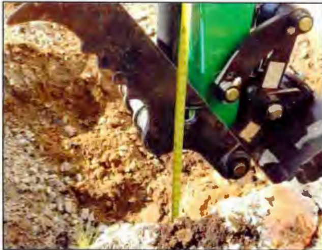
Photo 11. The upper 2.5 feet of soil was removed and placed on plastic to allow for treatment of the lower portion of soil. Extensive soil staining was present throughout the excavation. No odors were observed. [Photo taken looking south]
