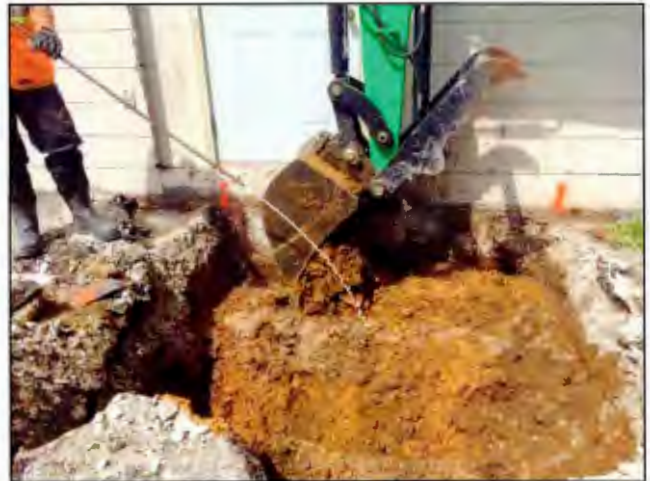
Photo 16. Cool-Ox™ was applied to the area of excavation and thoroughly blended with the lower three feet of soil using the bucket of the backhoe. The application rate of the solution was approximately ten gallons of solution per cubic yard. [Photo taken looking west]
