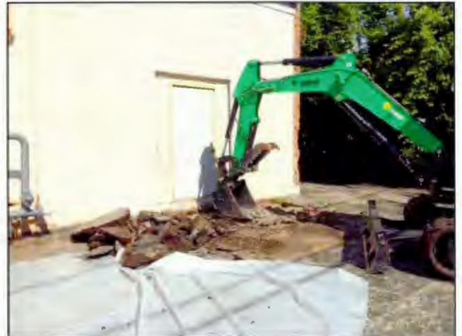
Photo 8. Excavated soil was maintained on plastic within the containment area until replaced and treated. [Photo taken looking northwest]
