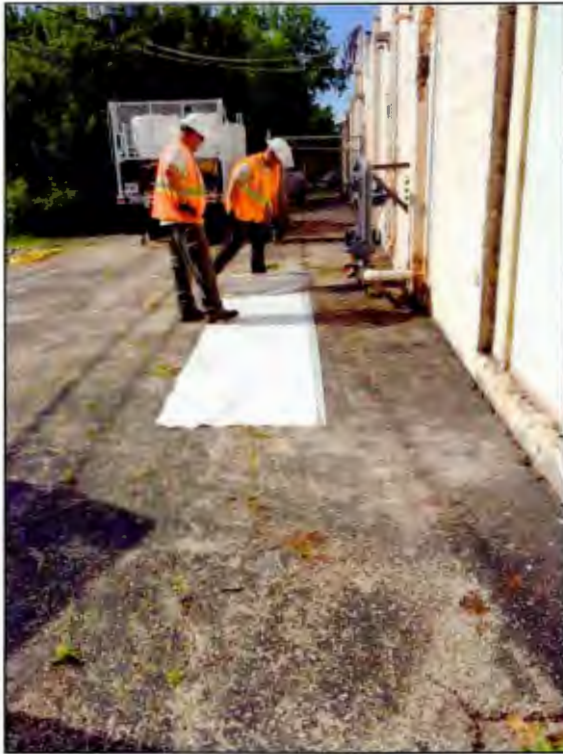
Photo 5. Plastic sheeting was placed near the area for piling excavated soil prior to remedial treatment. [Photo taken looking south]
