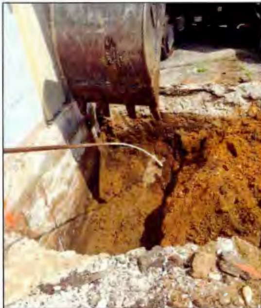
Photo 15. Soils were accessed to 5 feet (just above saturated soils). Using a Terracore™ sampler, a sample was collected from soils from the 4.5-ft depth from the backhoe bucket prior to applying the Cool-Ox™ treatment solution. [Photo taken looking northwest]
