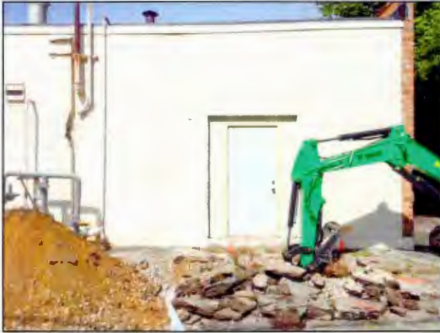
Photo 13. The remedial excavation was completed to 2.5 feet. Soil was piled on plastic south of the treatment area. [Photo taken looking west]
