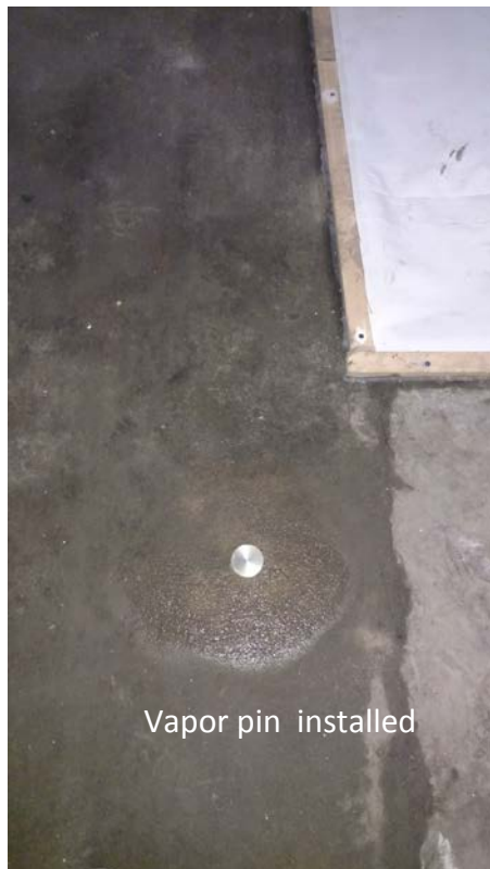
Floor area near crawl space sealed with mortar in large joints and polyethylene caulk in smaller joints
