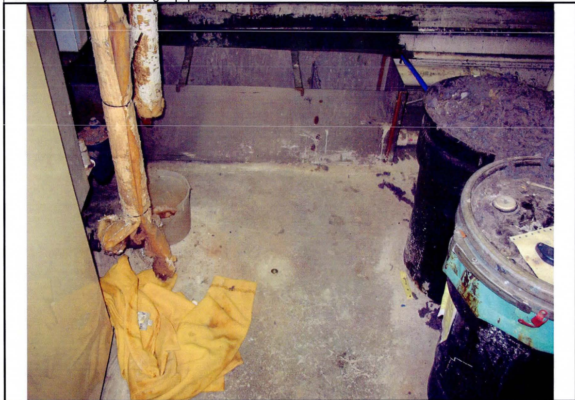
2. View of the flush-mount gas vapor sampling point to the north of the dry cleaning equipment.
