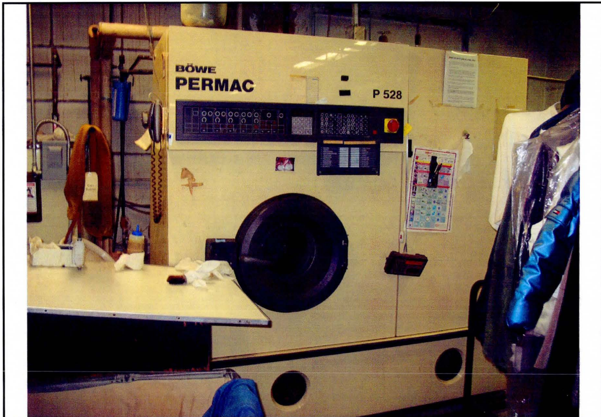
1. View of the dry cleaning equipment inside One Hour Fabricare.
