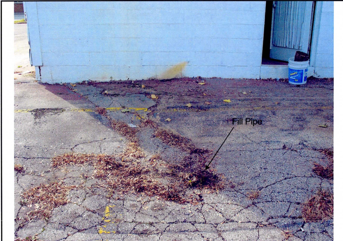
15. View of the fill pipe to the underground storage tank to the north of the dry cleaning building.
