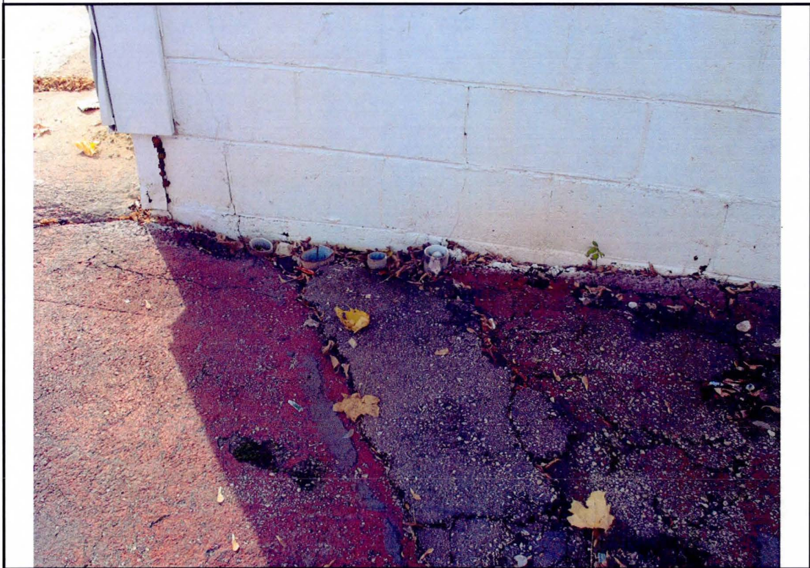
16. View of pipes adjacent to the north side of the dry cleaning building.
