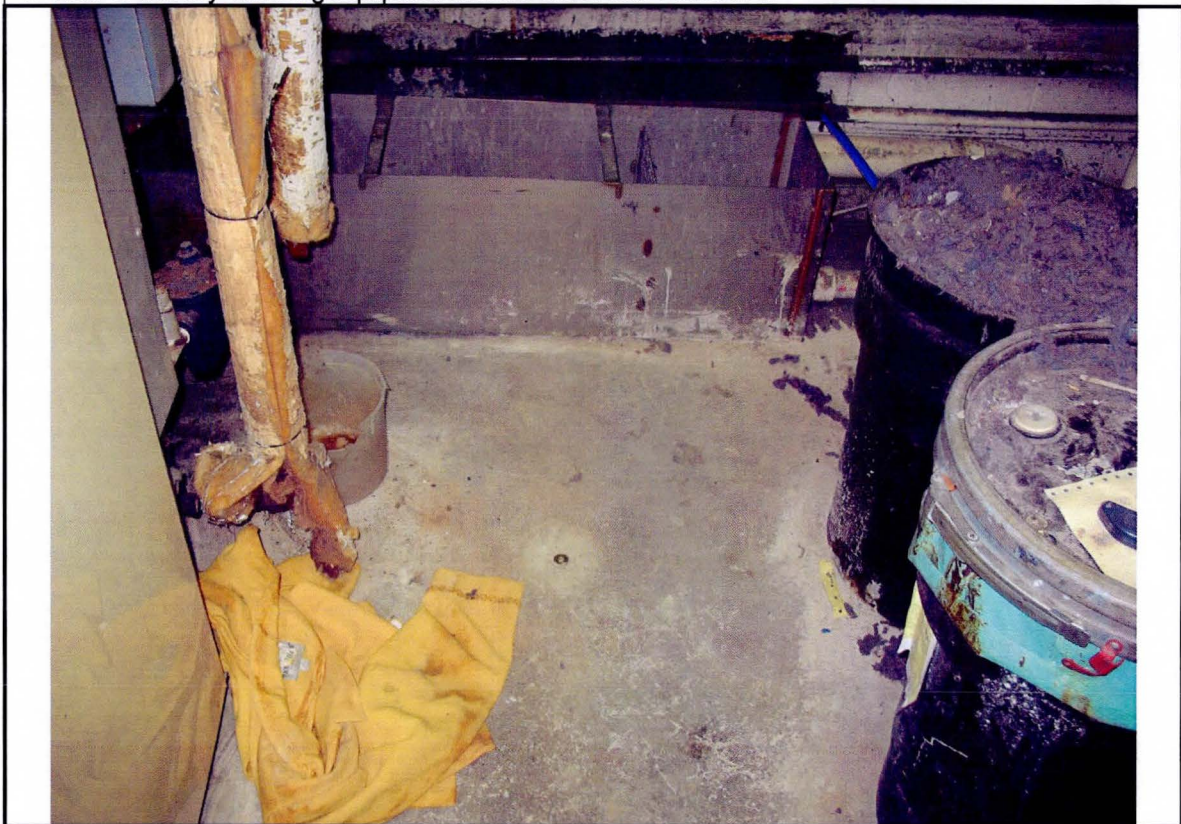
2. View of the flush-mount gas vapor sampling point to the north of the dry cleaning equipment.
