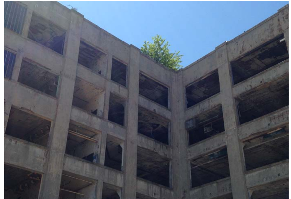
Windows removed and openings left; not weather-proof.
