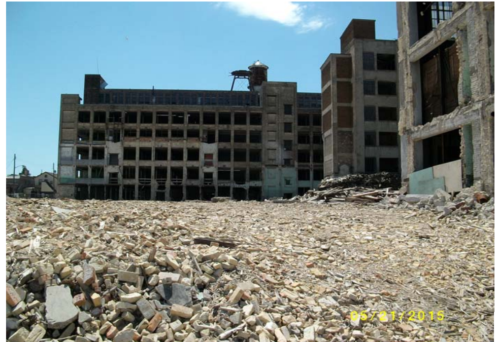
Demolition materials left on site.
