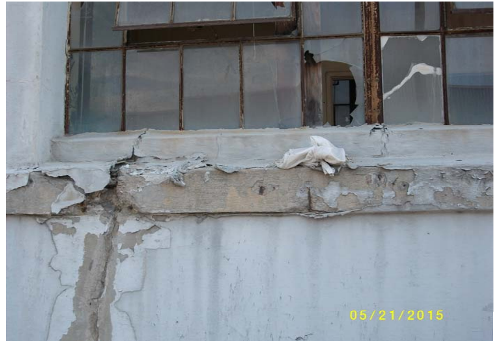
Crumbling building exterior; hazardous materials on site (asbestos).
