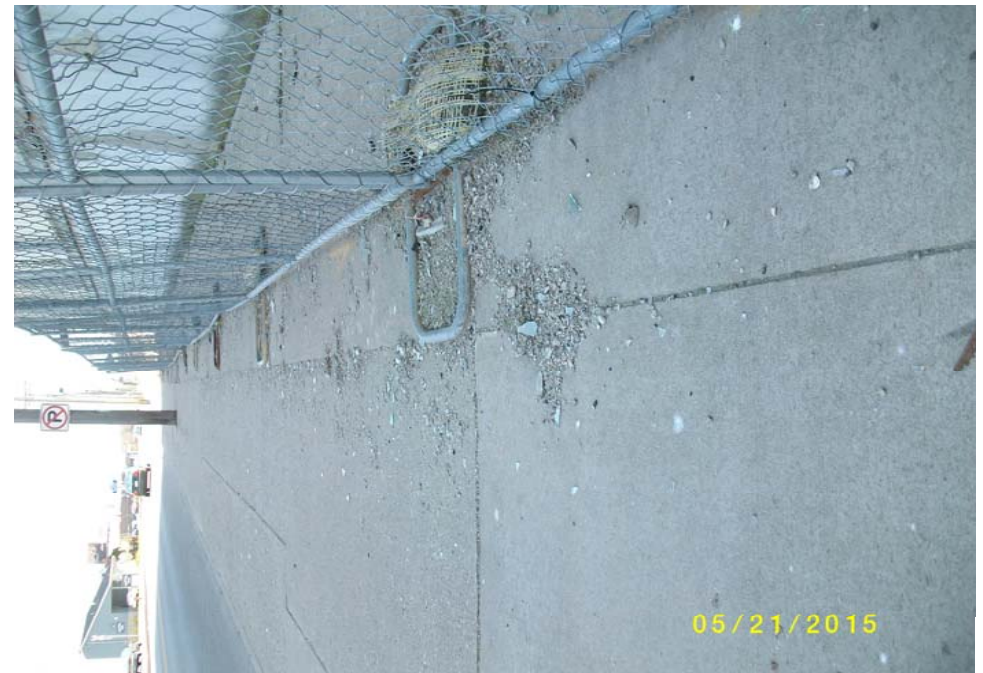
Various building materials crumbling onto sidewalk.
