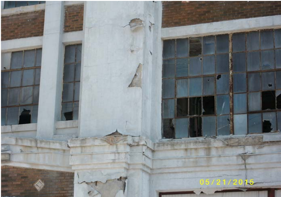
Crumbling building exterior; damaged windows.
