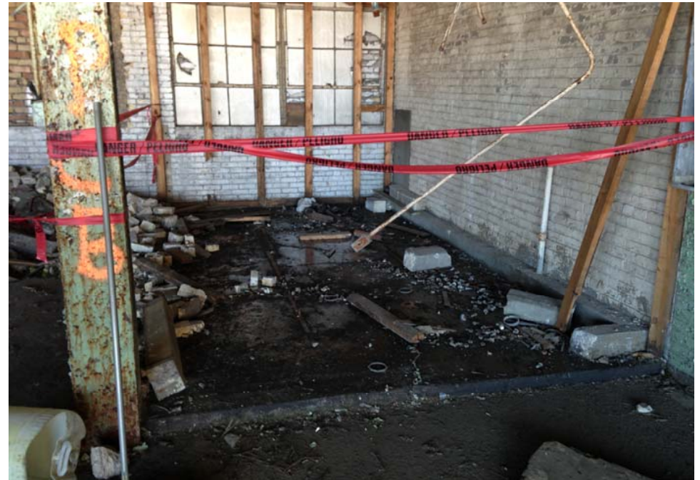
PCB oil spill.
