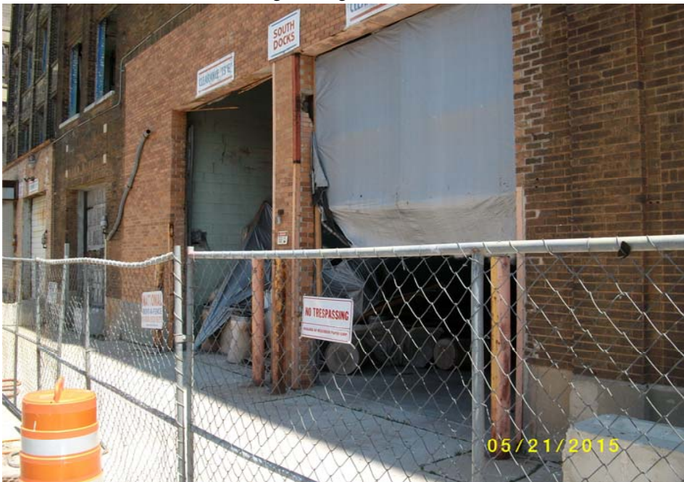
Torn and falling down tarps left on site.
