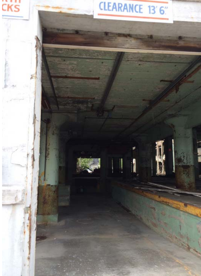
#17 - View of N loading dock and bldg interior, looking east from 16th St
