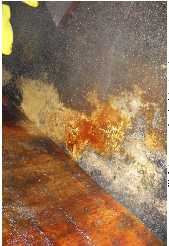
#28 - Stained concrete wall and floor in tunnel network
