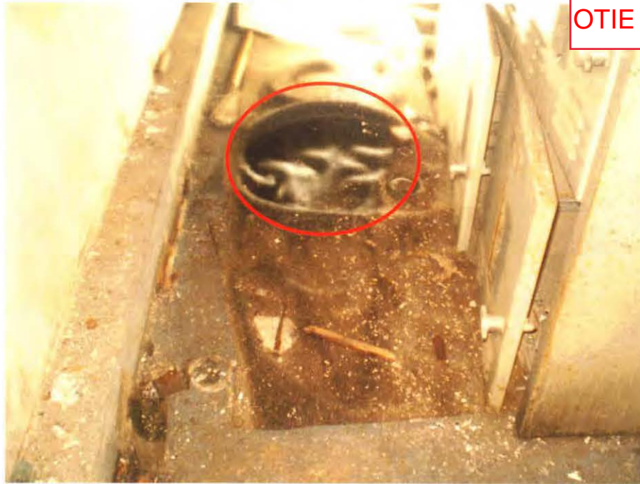
Photograph No.: 11 Photographer: Caitlin Ruza Area: Bldg I-Transformer TDD Number: TO-05-10-12-0002 Contract: EP-S5-10-10, OTIE Date: January 24, 2011 Site Name & Location: Mirro-Spirtas Site, Manitowoc, Manitowoc County, Wisconsin Photograph Subject: MS-WP-6 collected from puddle on plastic matting in the transformer room in Building I (approximate sample area shown)
