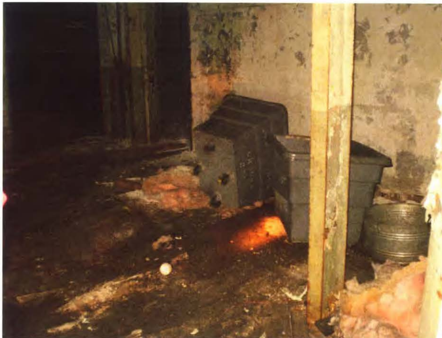
Photograph No.: 2 Photographer: Caitlin Ruza Area: Bldg K-Loading Dock TDD Number: TO-05-10-12-0002 Contract: EP-S5-10-10, OTIE Date: January 24, 2011 Site Name & Location: Mirro-Spirtas Site, Manitowoc, Manitowoc County, Wisconsin Photograph Subject: Two wheeled bins in the loading dock area of Building K. One bin is tipped over and one contains the contents which has been drained from the transformer on the second floor above
