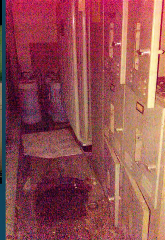
Photos of PCB Transformer Room, Building I (aka Area 8), during site walkthroughs:
