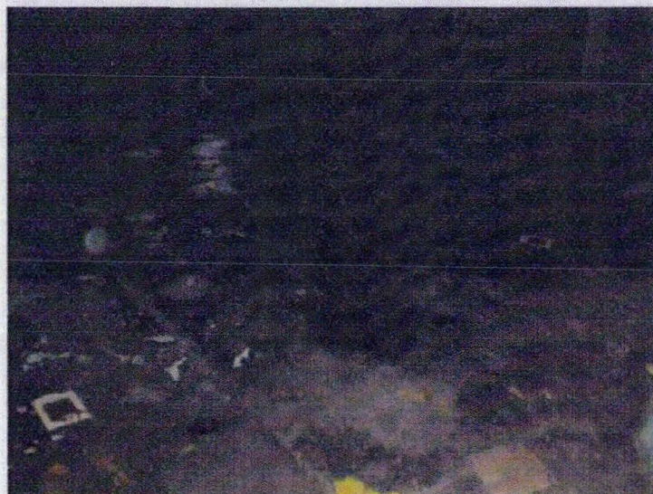
PCB contaminated floor; transformer oil spillage area
