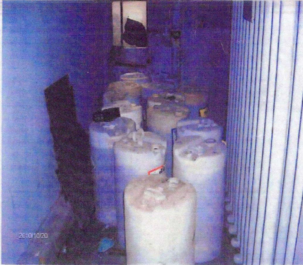
Drums containing transformer oil at Mirro Spirtas Site
