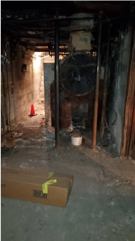
Photo 3: Basement – Looking north into adjoining basement of 616 Oak Street, unused coal furnace shown.
