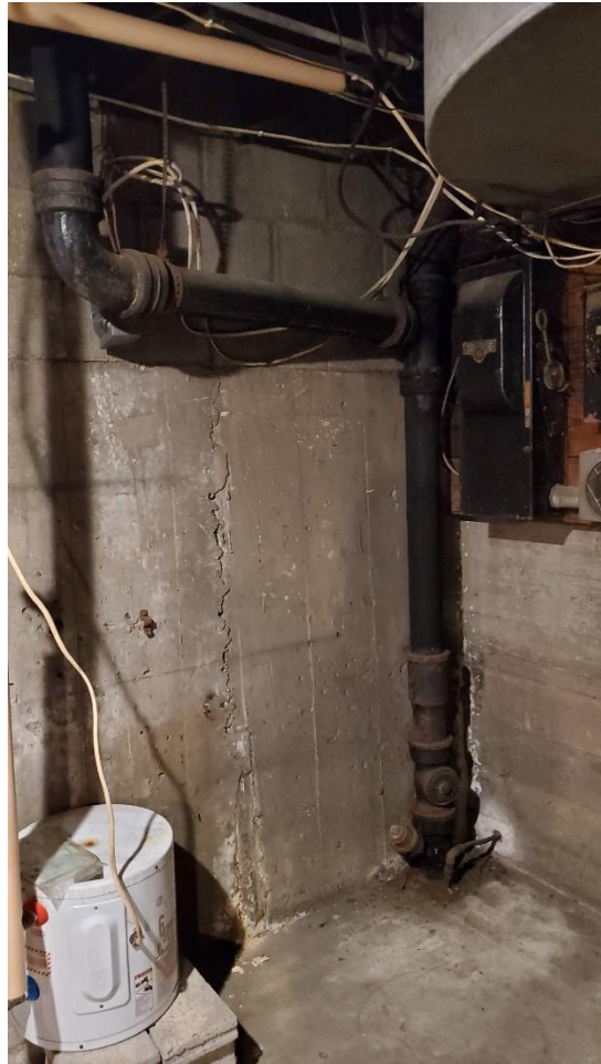
Photo 4: Basement- Northeast corner of basement. Plumbing stack, electric water heater, and electrical panel shown. Minor cracking along concrete forms shown.
