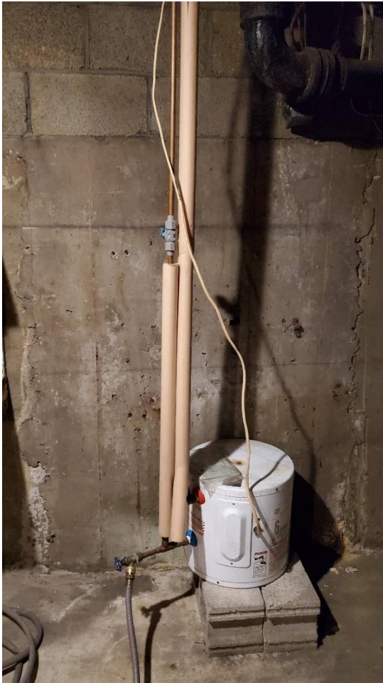
Photo 7: Second view of the basement-Electric water heater, and minor cracking along concrete forms, and transition from poured wall to blocks shown.
