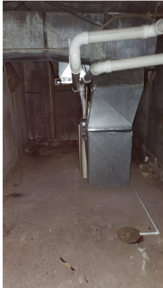
Photo 2: Basement- West end of the basement looking south. The furnace and floor drain is shown.
