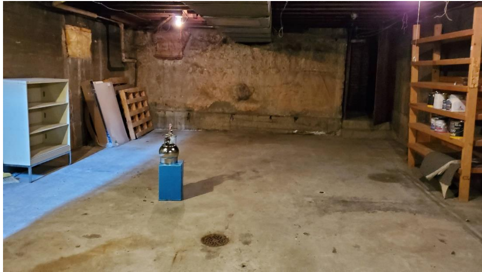
Photo 5: Basement view to the west- Wall separating furnace room and floor drain shown. Likely window well on left side (south wall along alley) with insulation also shown.
