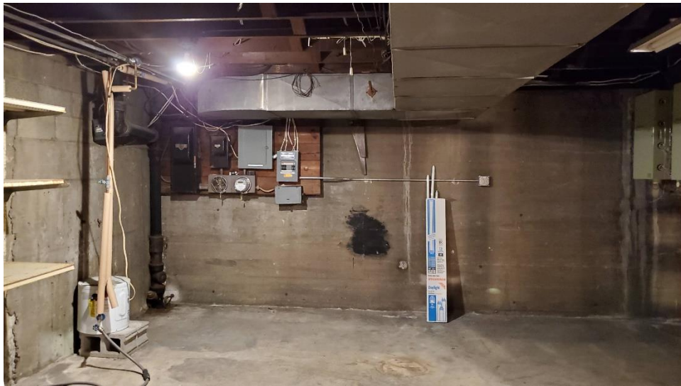
Photo 6: East basement wall, plumbing stack, electrical panel, water heater, and HVAC duct work shown.
