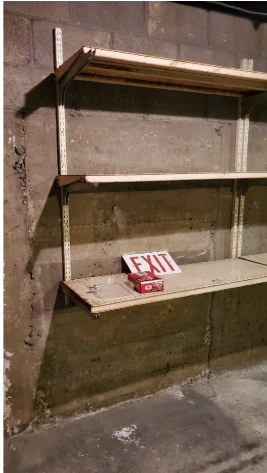
Photo 8: North basement wall, west of Photo 7, minor cracking along concrete forms, and transition from poured wall to blocks shown.
