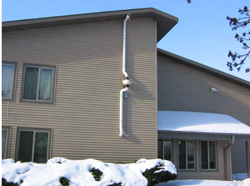
Photo 2: View of the vapor vent system on the 1003 building
