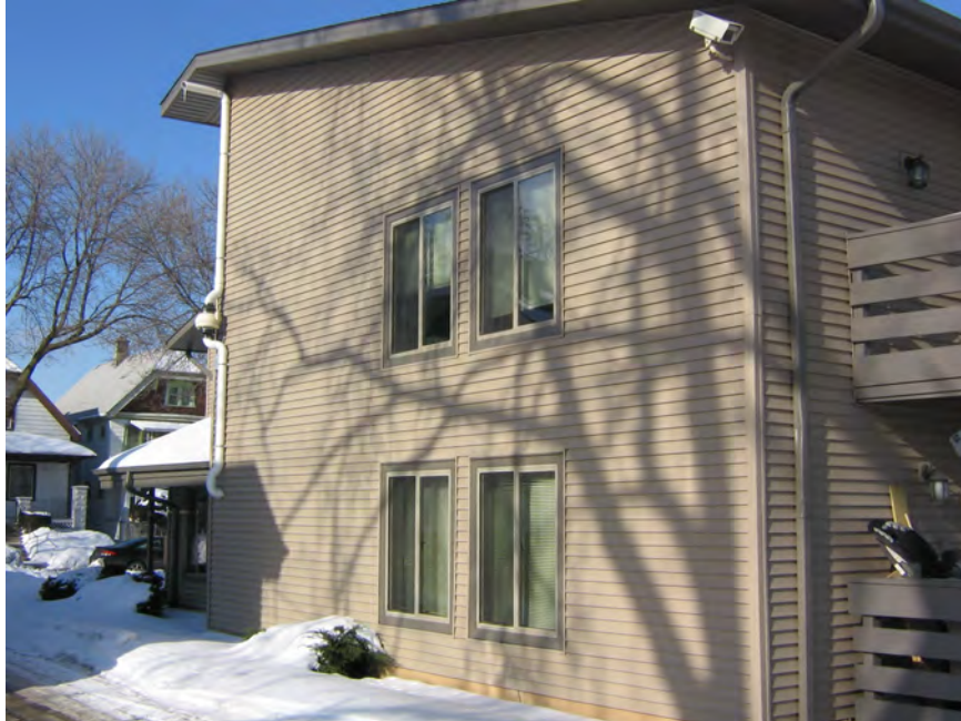
Photo 4: View of the vapor vent system on the east 1033 building
