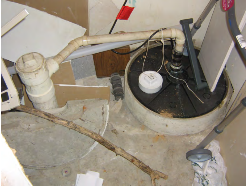
Photo 5: View of the sump system located in each of the apartment buildings
