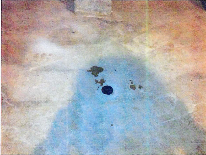
Photo 5: 2/6/2014 – Photograph of capped sub-slab vapor probe in basement of home.
