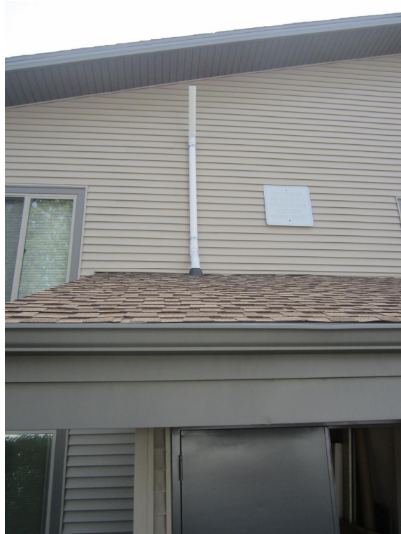
Photograph looking east at 1003 West Atkinson Shed SSSS exterior piping on west side of building.
