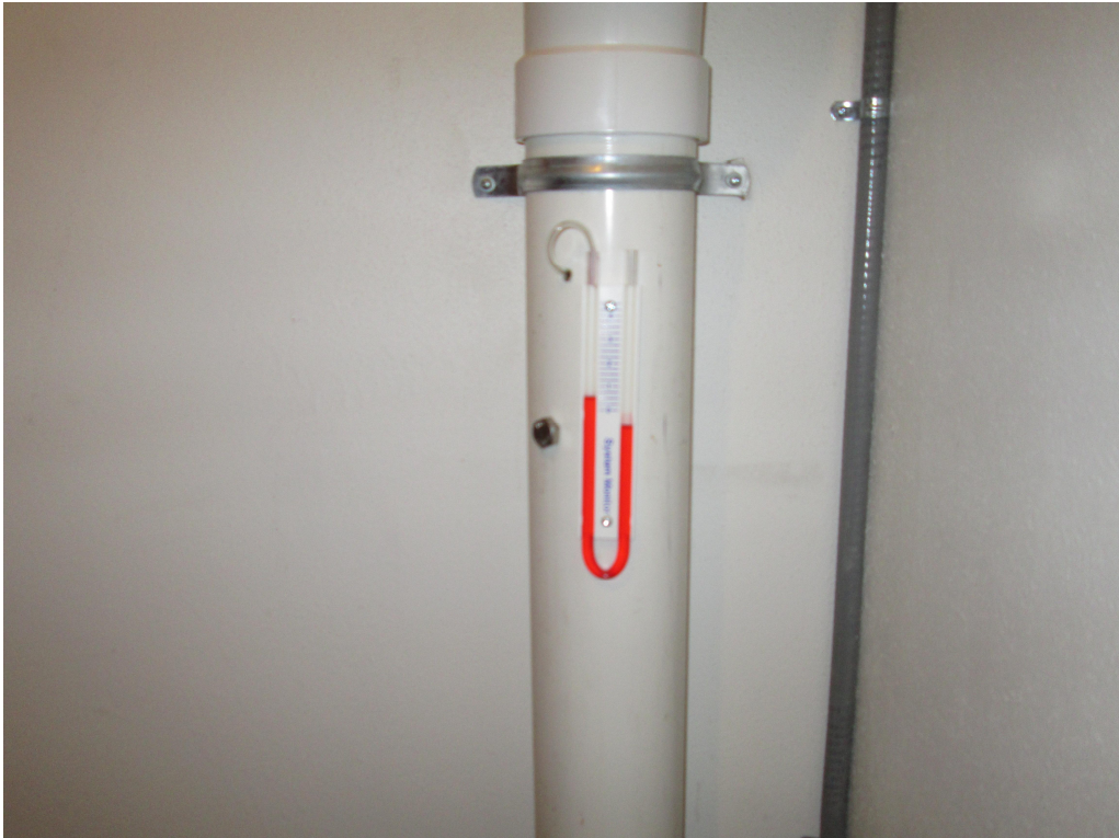
Photograph looking at 1033 West Atkinson Closet SSDS manometer.
