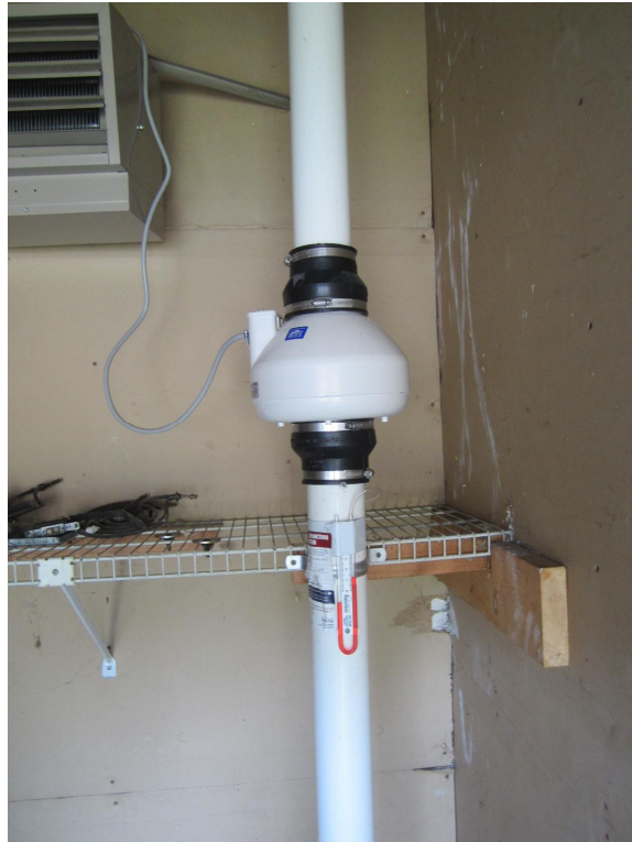
Photograph looking at 1033 West Atkinson Shed SSDS manometer.
