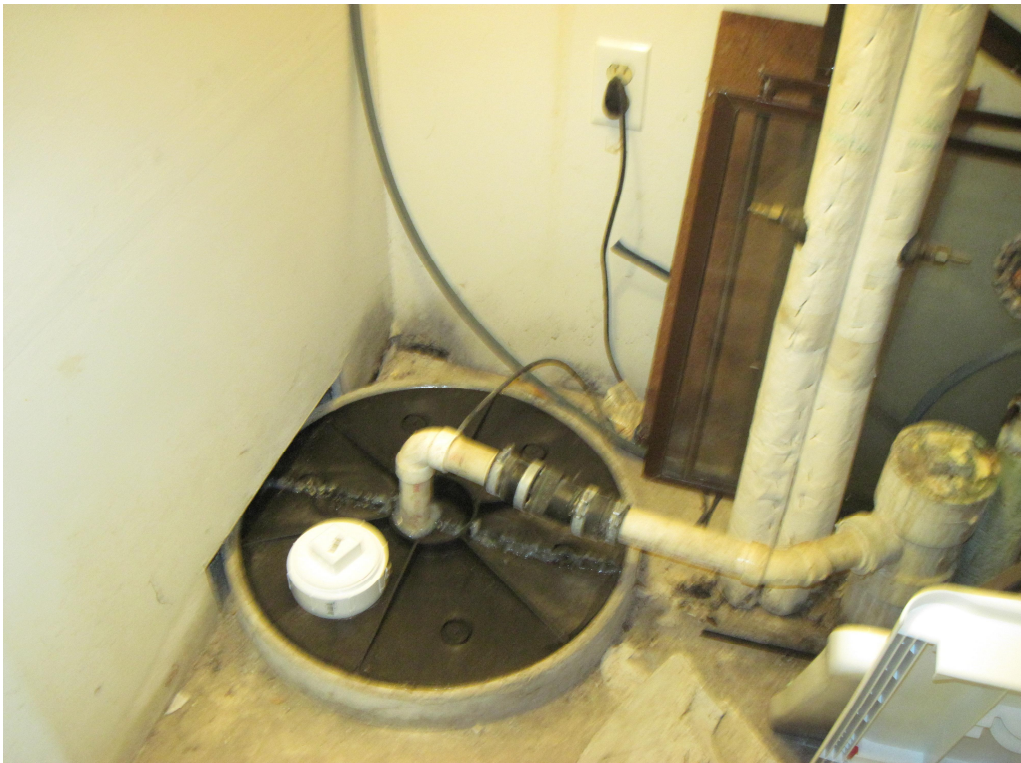
Photograph looking at 1033 West Atkinson sealed sump located across the hall from elevator.
