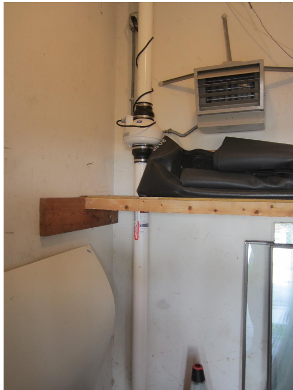
Photograph looking at SSSS system inside 1003 West Atkinson shed located on west side of building.
