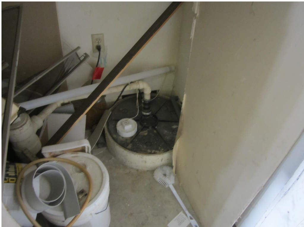
Photograph looking at 1003 West Atkinson sealed sump located across the hall from the elevator.
