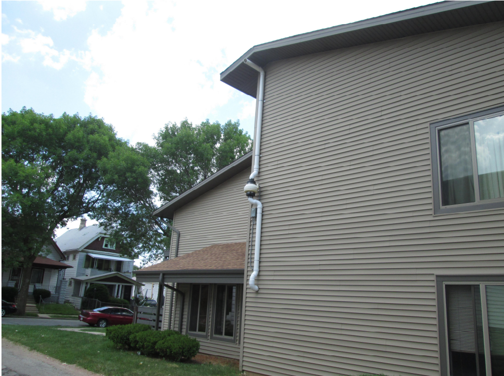
Photograph looking west at 1033 West Atkinson Closet SSDS system and exterior piping on south side of building.
