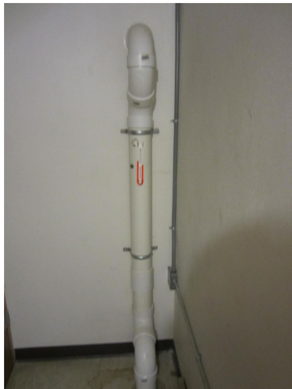
Photograph looking at SSDS system piping inside 1033 West Atkinson closet located in south side of building.
