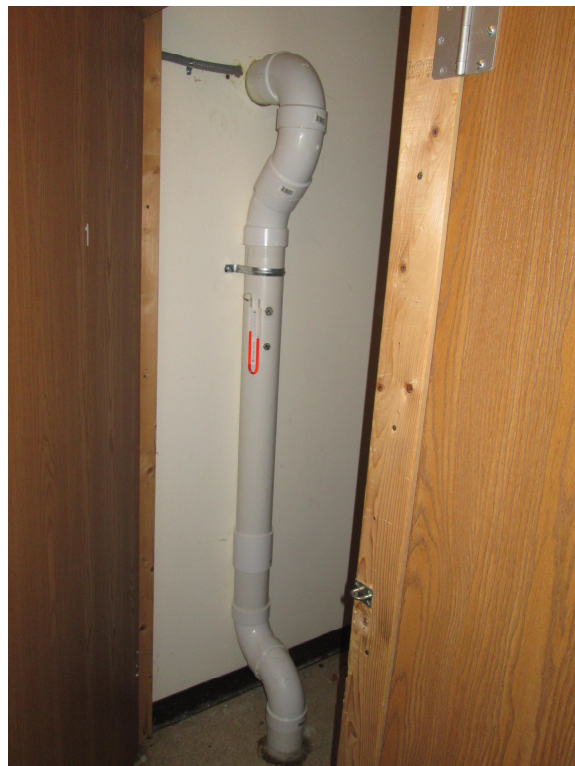
Photograph looking at SSDS system inside 1003 West Atkinson closet located inside the east side of building.
