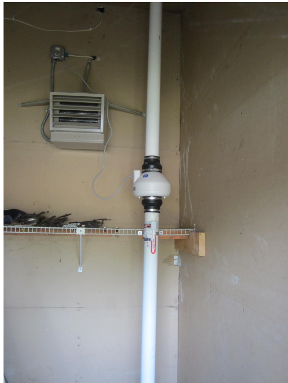
Photograph looking at SSSD system inside 1033 West Atkinson shed located on north side of building.
