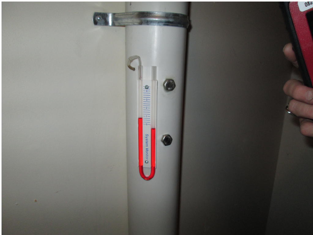
Photograph looking at 1003 West Atkinson closet SSDS manometer located in east side of building.
