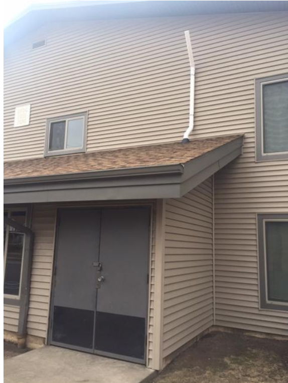
Photograph looking south at 1033 West Atkinson Shed SSSD exterior piping on north side of building.
