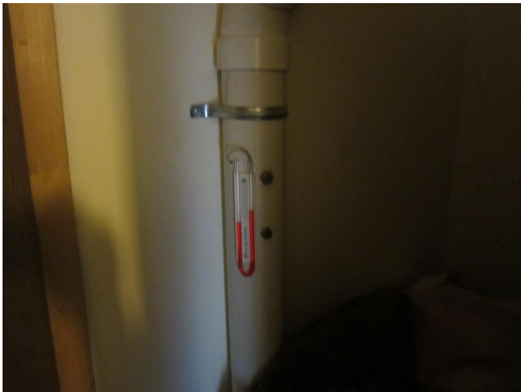
Photograph looking at 1003 West Atkinson Shed SSDS manometer.
