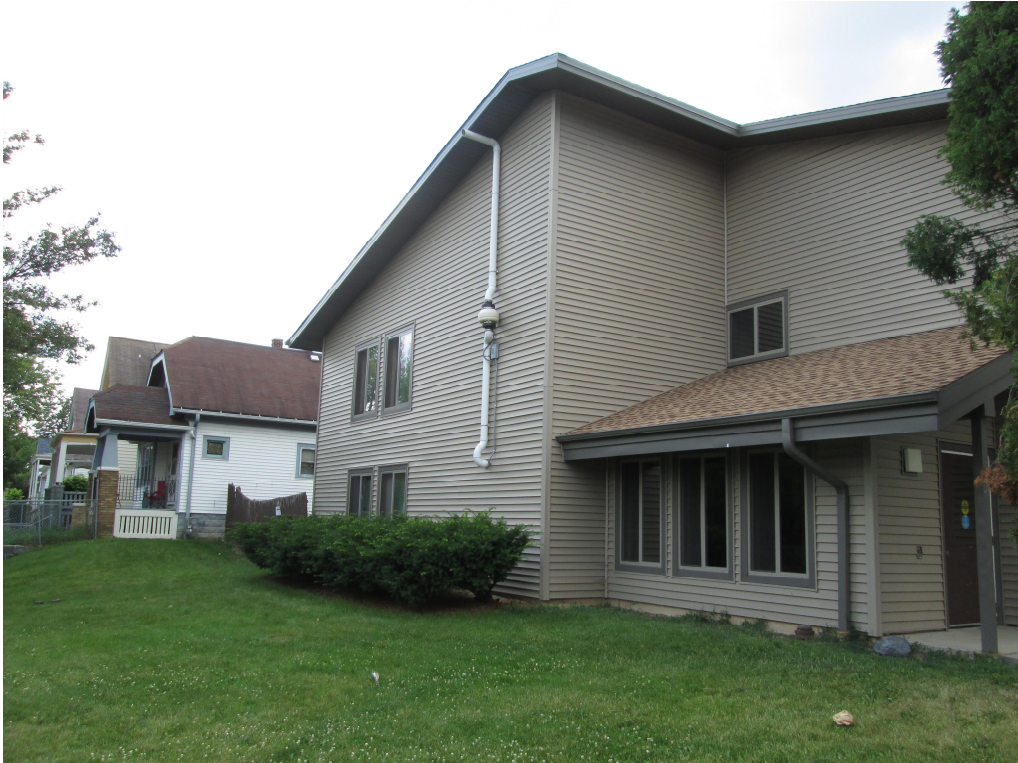
Photograph looking south at 1003 West Atkinson Closet SSDS exterior piping on east side of building.
