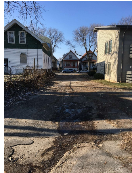
Looking to the west along alley, catch basin located at end of alley
