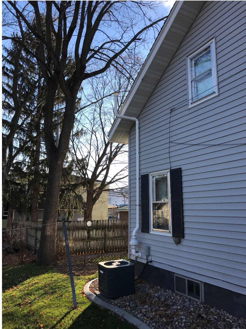
Photo 9: Blower and exhaust line. November 30, 2021.
