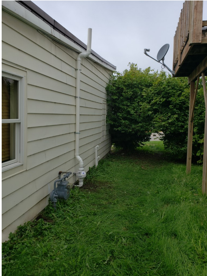
Photo 8: Blower and exhaust line. August 31, 2021.
