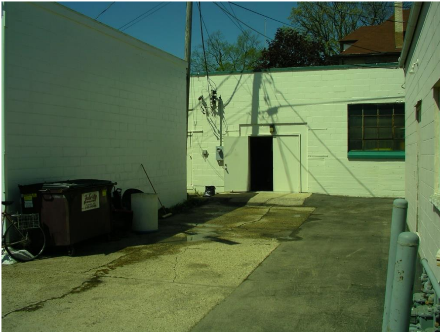
Photo 4: Northeast end of the Platteville Cleaners property, capped with concrete and asphalt.
