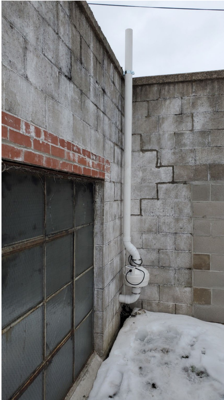
Photo 4: Fan and Exhaust Piping. January 31, 2024.
