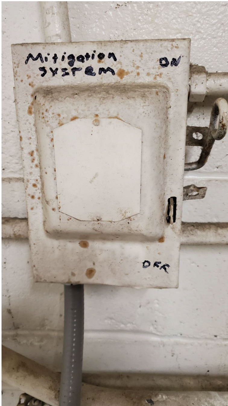
Photo 9: Fan On/Off Switch. February 21, 2024.
