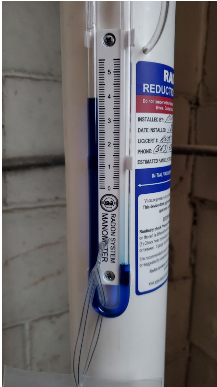
Photo 2: Pickup Point 1 manometer. January 31, 2024.
