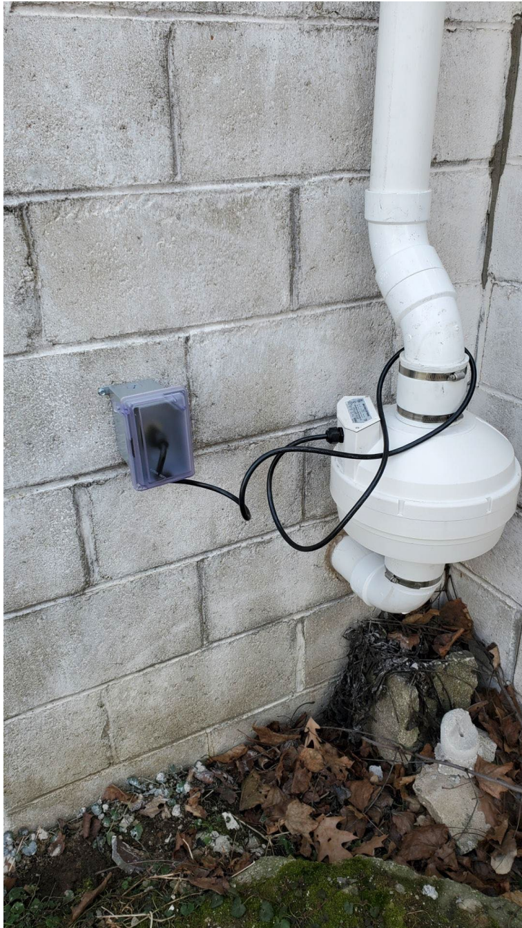
Photo 8: Fan Electrical Connection. February 21, 2024.
