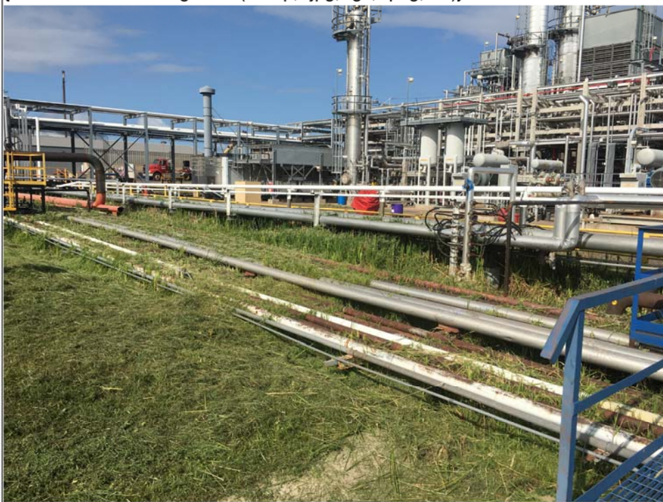
Title: Spill area under structural impediment (piping), green gas unit in background. Viewing NW.
