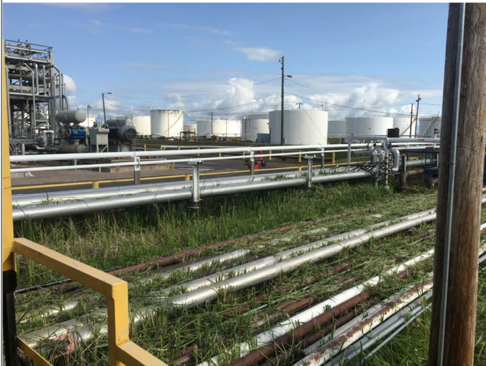
Title: Spill area under structural impediment (piping), SE corner of green gas unit in upper left. Viewing NE.
