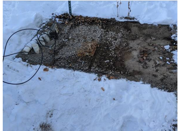
Photo #2 Photograph of SVE system component locations after removal.
