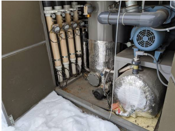
Photo #1 Photograph of SVE system before removal.
