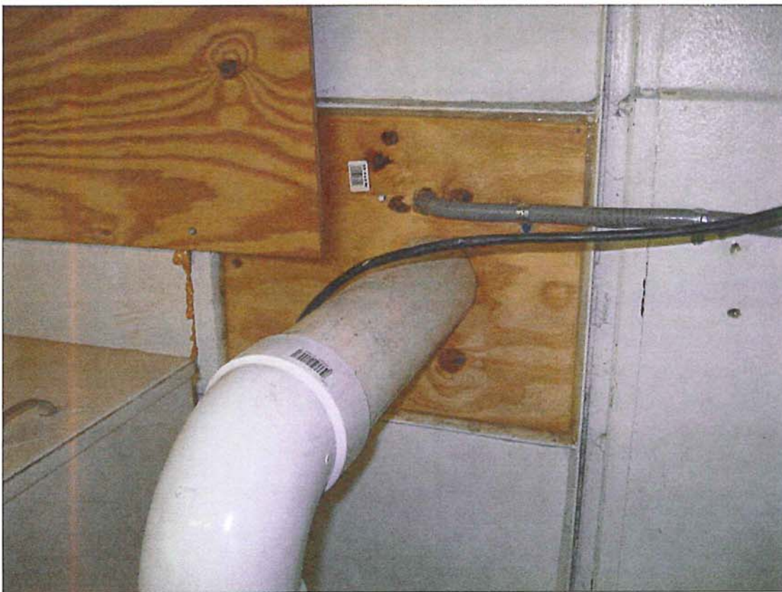
Photograph #: 2 Date: 5/24/2011 Direction: Inside site building Subject: Exhaust pipe exiting building
