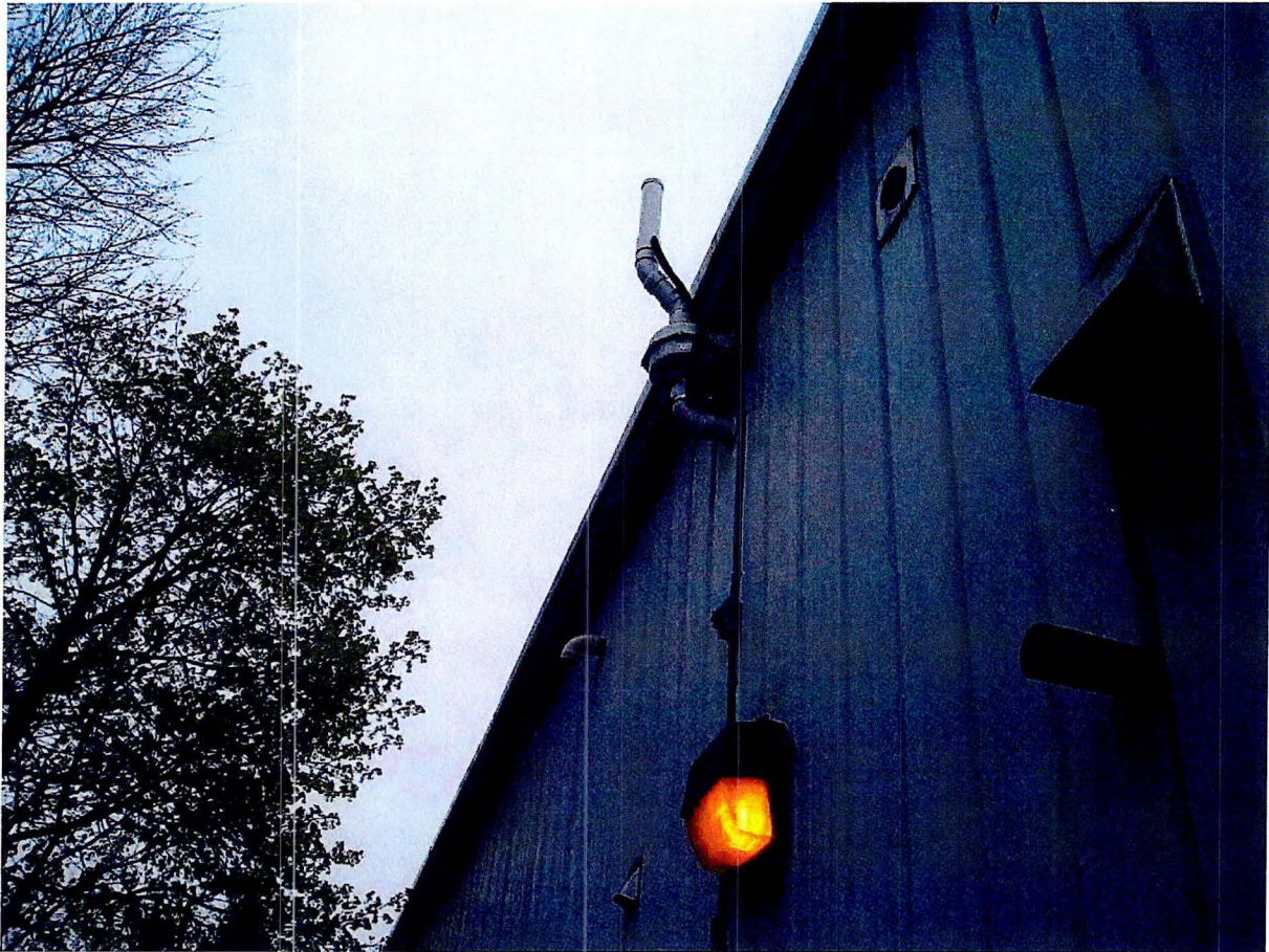
Photograph 2: VMS Fan, Electrical Switch and Exhaust. May 3, 2013
