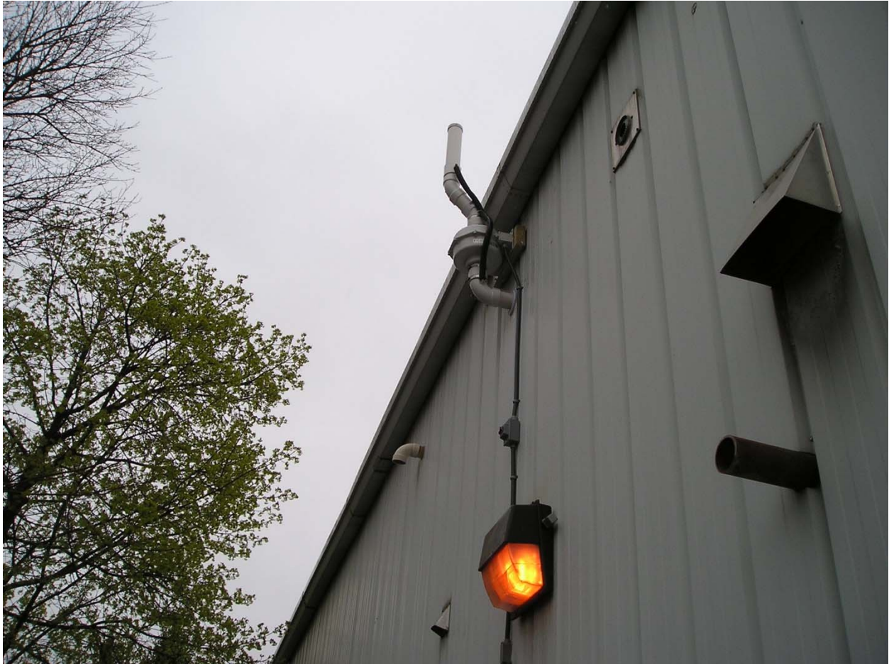
Photograph 2: VMS Fan, Electrical Switch and Exhaust. May 3, 2013
