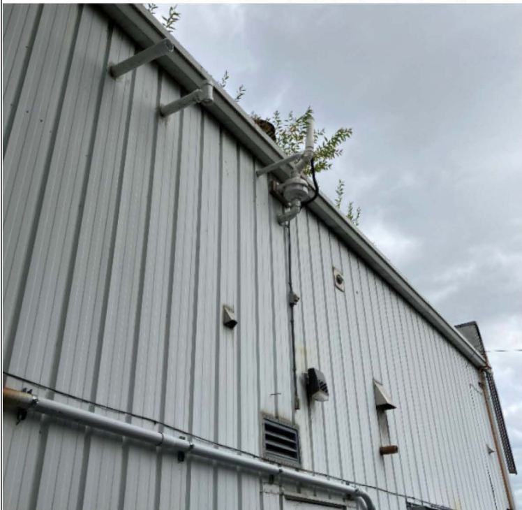
Title: View of VMS exhaust on south side of building
