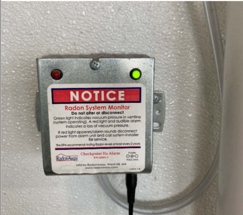
Title: VMS system alarm box
