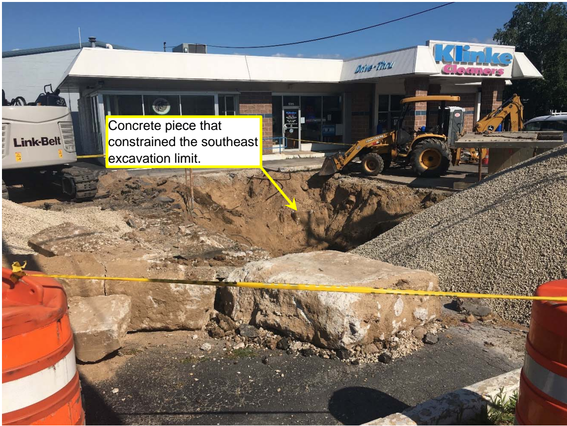
Excavation overview, facing southeast. The concrete slabs in the foreground were removed from the west side of the excavation.
