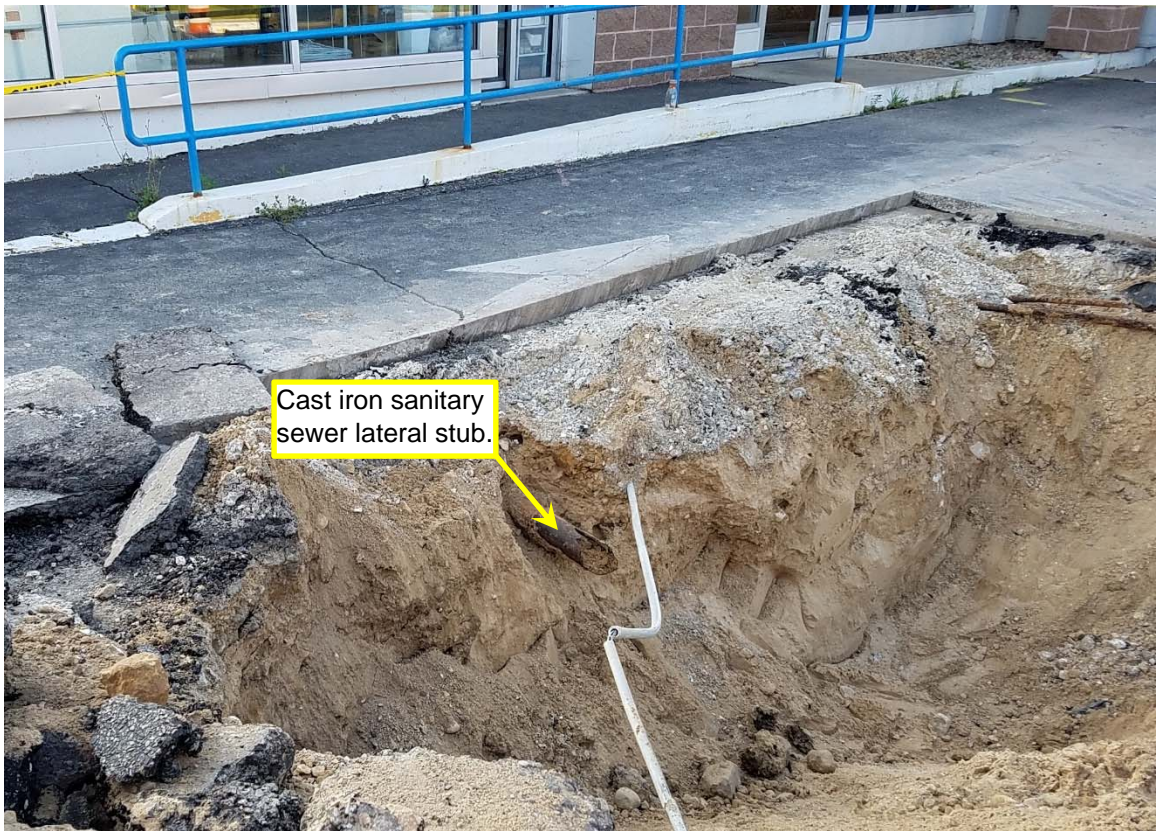
East side of excavation showing the sanitary lateral stub to which new PVC pipe was connected.
