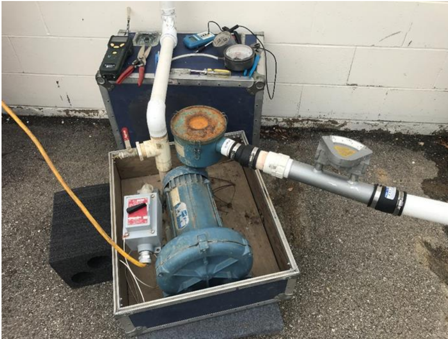
Photo 5: SVE pilot test blower, flowmeter, and discharge piping. August 13, 2019.
