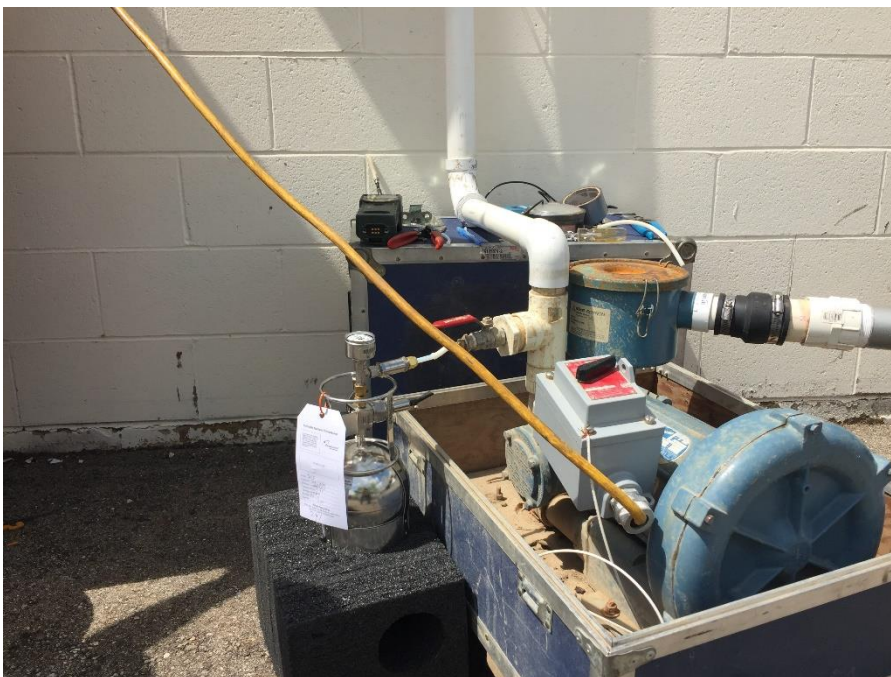
Photo 6: SVE blower and summa canister for sampling exhaust air. August 13, 2019.
