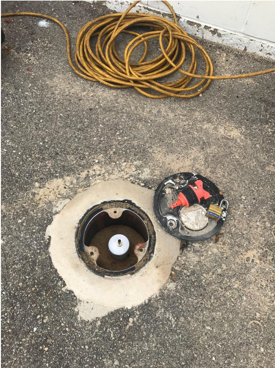
Photo 4: SVE well with slip cap and barb fitting for vacuum measurements. August 13, 2019.
