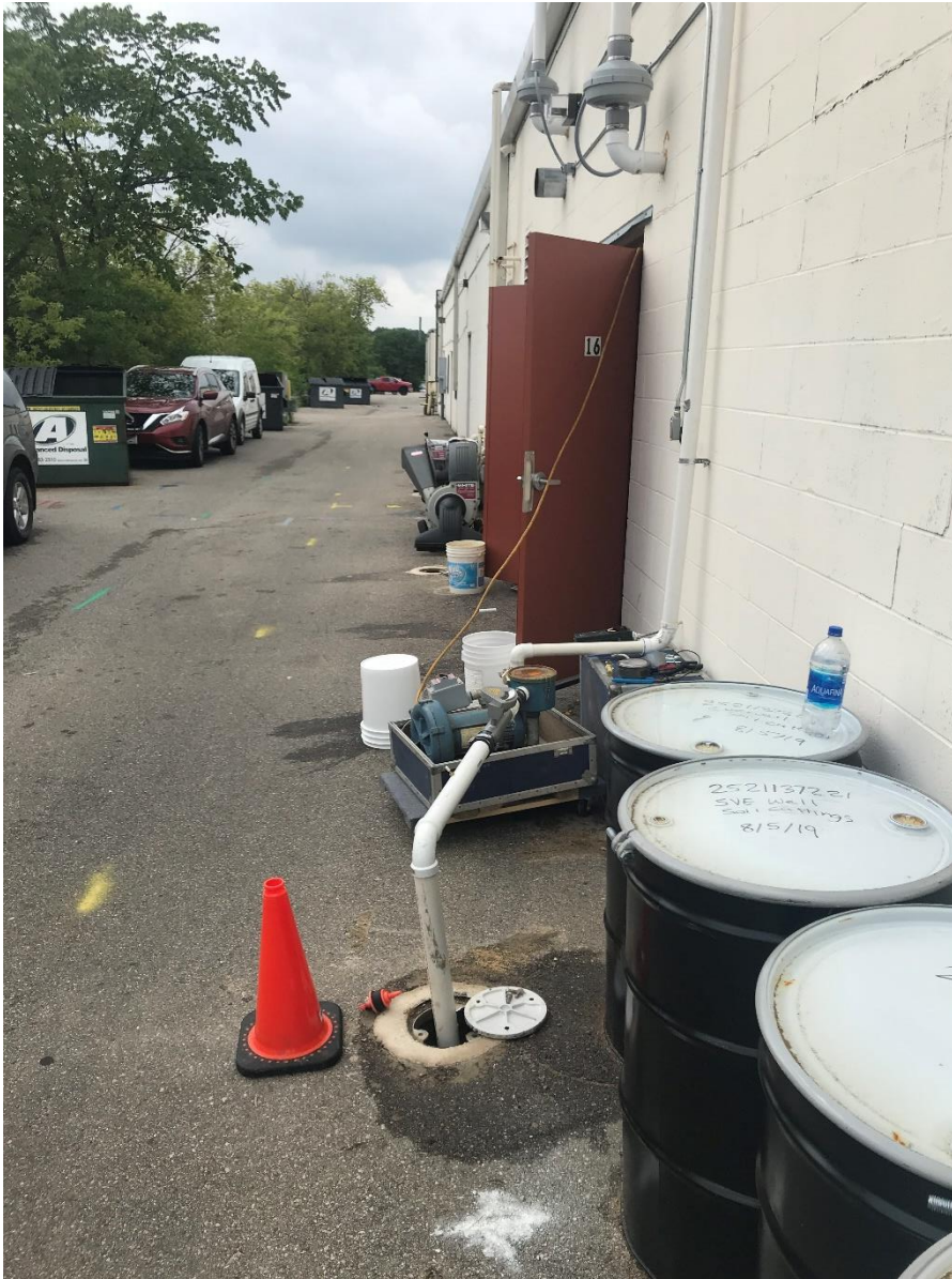
Photo 7: SVE pilot test blower setup showing SVE well SVE1, SVE blower, piping. August 13, 2019.
