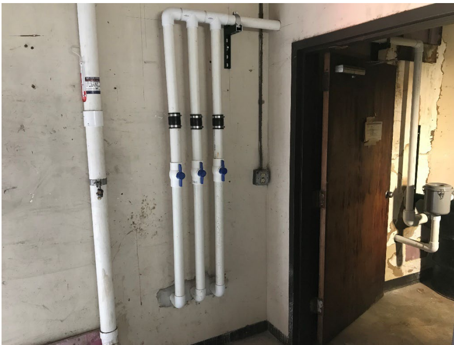
Photo 6: SVE piping and valves inside building. Date: 9/13/22 Photo direction: East
