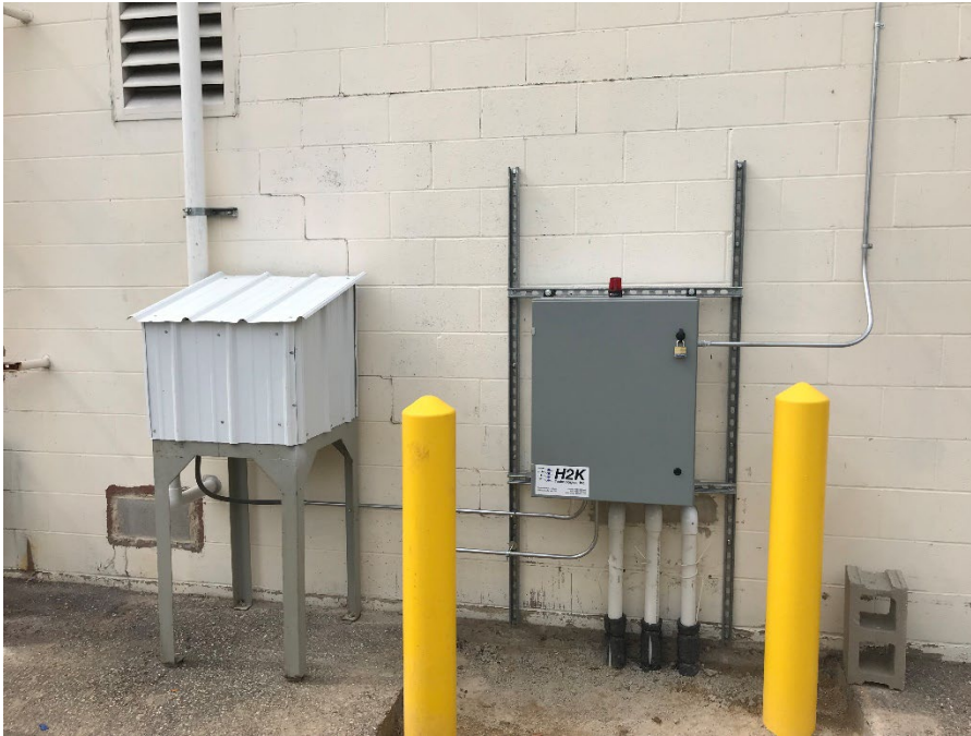
Photo 9: SVE system control panel (right) and SVE blower inside sheet metal enclosure (left). Date: 9/21/22 Photo direction: west
