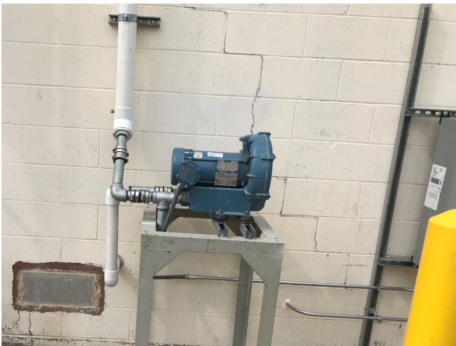
Photo 8: SVE blower and SVE piping. Date: 9/21/22 Photo direction: west
