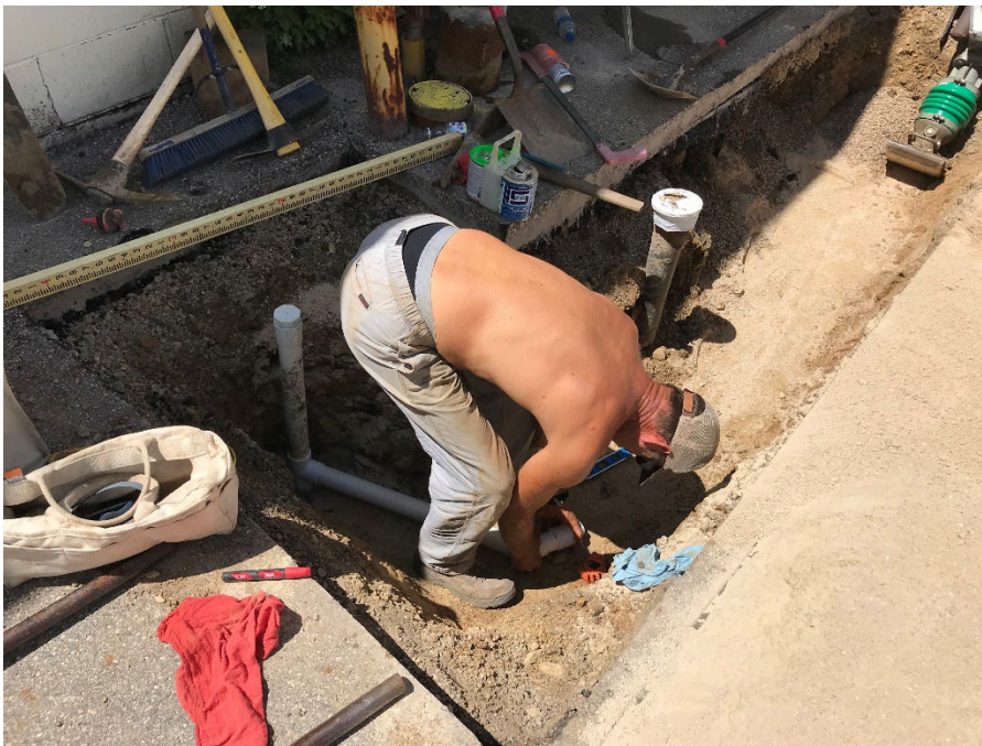
Photo 2: Installing 2-inch diameter PVC piping to SVE well SVE-3. Date: 7/28/22 Photo Direction: Northwest
