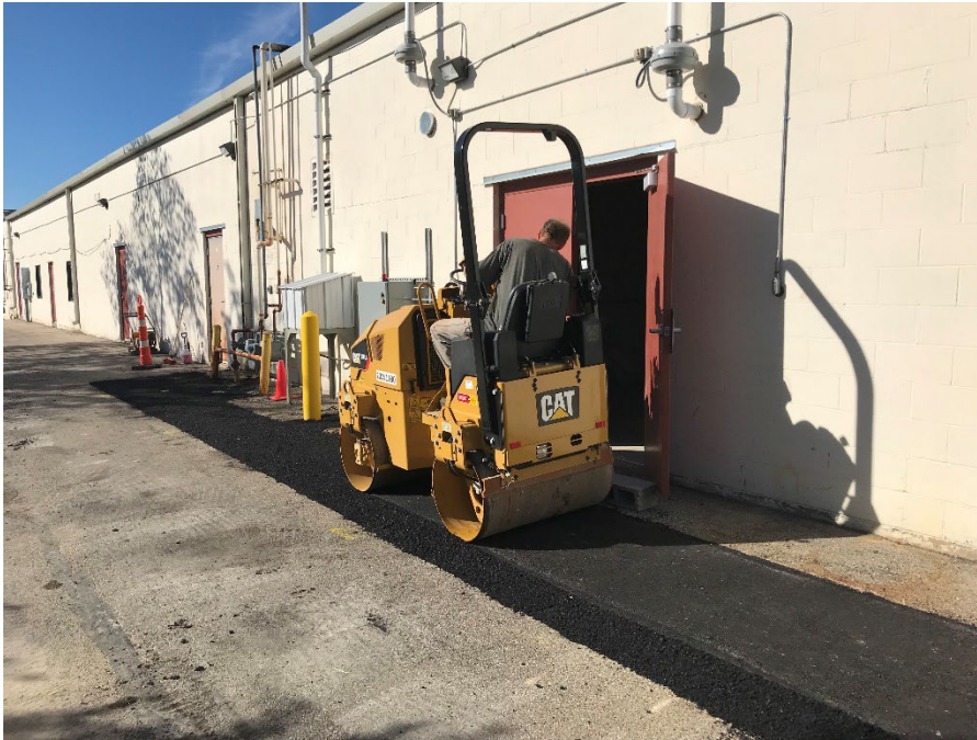
Photo 11: Compacting wearing asphalt in SVE trench using smooth drum roller compactor. Date: 9/29/22 Photo direction: Southwest
