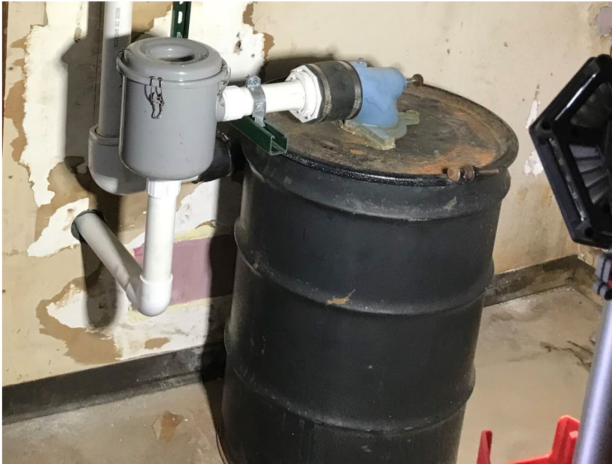
Photo 7: Air filter, knockout tank and SVE piping inside building. Date: 9/13/22 Photo direction: East
