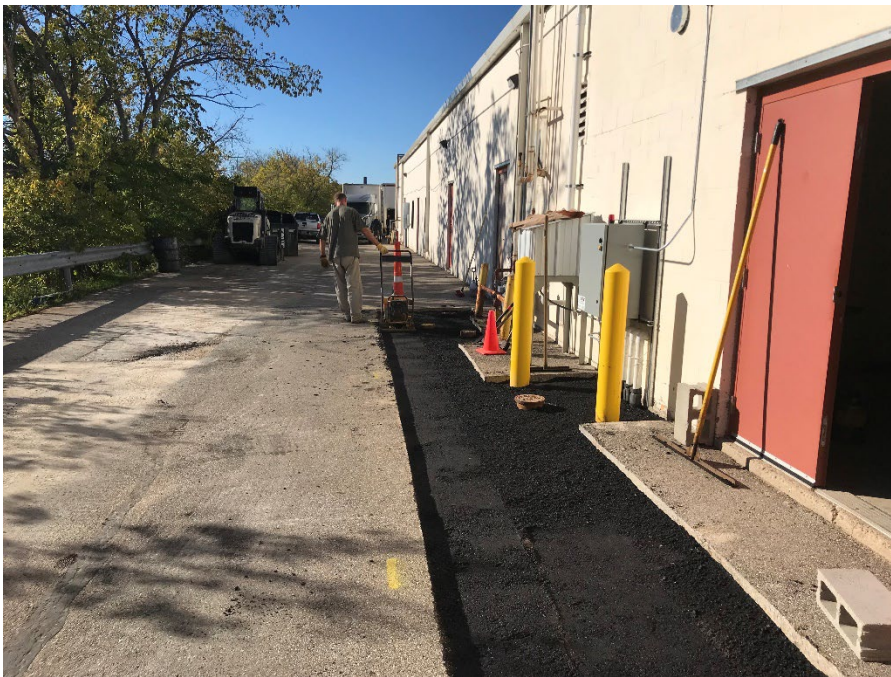
Photo 10: Compacting base course of asphalt in SVE piping trench using plate compactor. Date: 9/29/22 Photo direction: South
