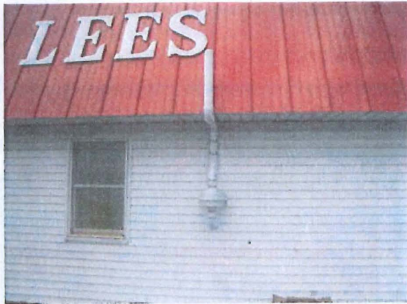
South fan outside Lee's Cleaners building. Looking north.
