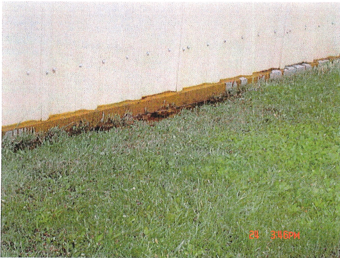
Spilled liquid seeped onto grass and flowed to swale
