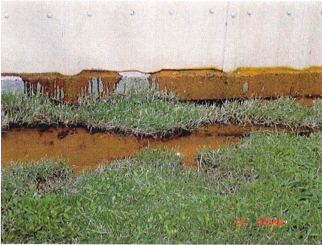
Acid seeping under building wall and onto grass
