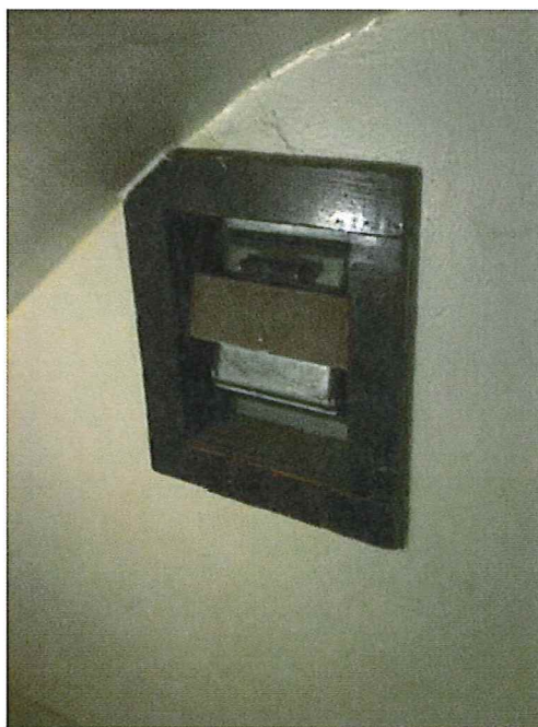
Sealed incinerator chute
