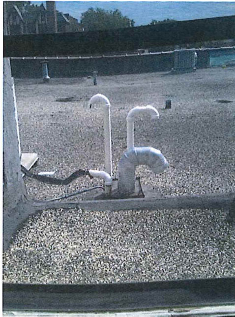
Fresh air intake
