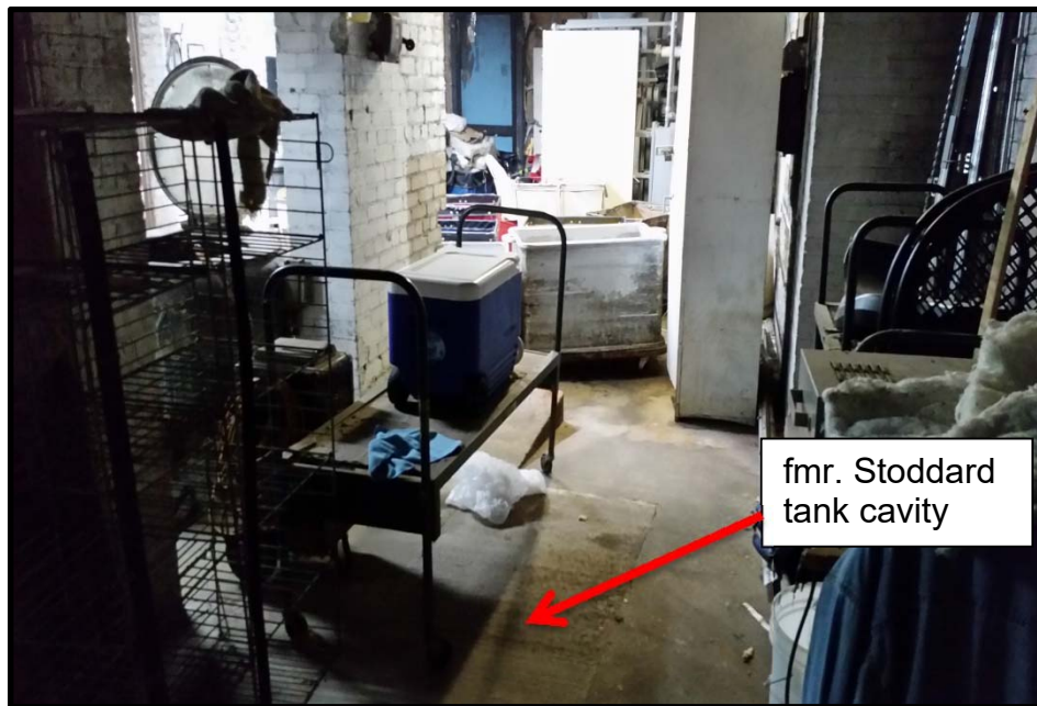
Photo 4 – This photograph looks north from the vantage of the exterior door shown in photo 1. The different concrete shown in the foreground is evidence of the former location of the Stoddard tanks.
