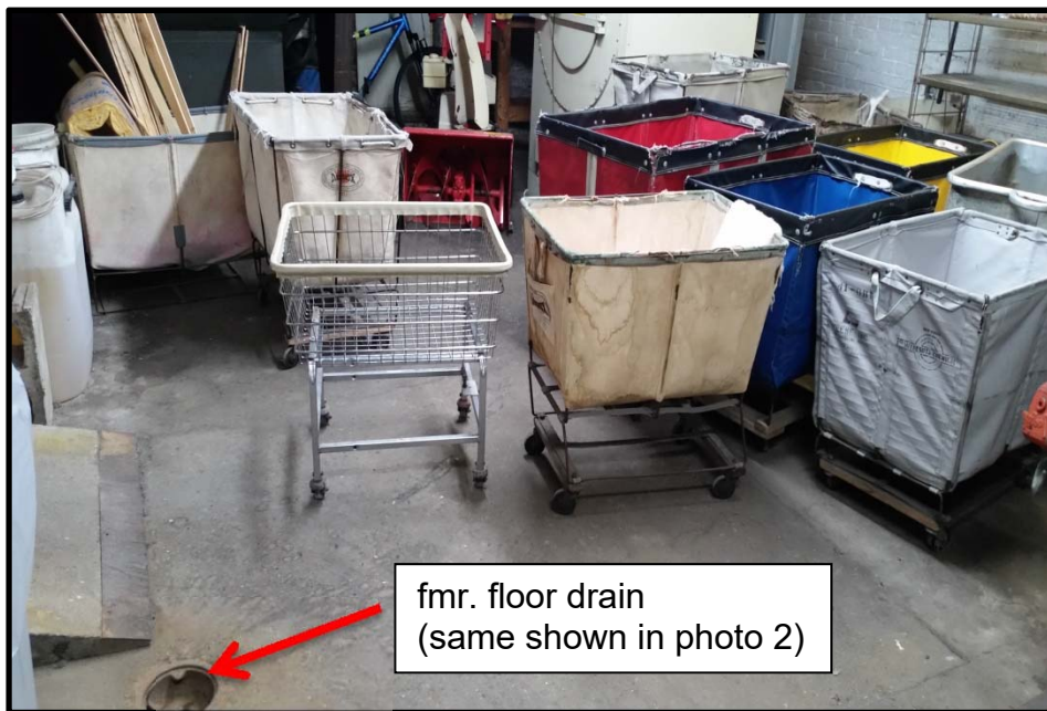
Photo 3 – This photograph shows another vantage of the floor drain shown in the previous photo.
