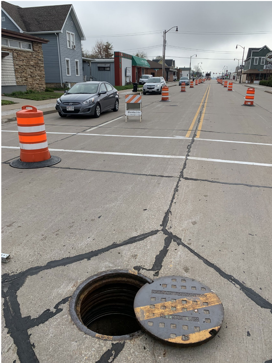
Photo 1: Looking east down W. Wisconsin Ave with sanitary manhole “SAN MH 58-24” in the foreground. Traffic control measures are shown in the background.
