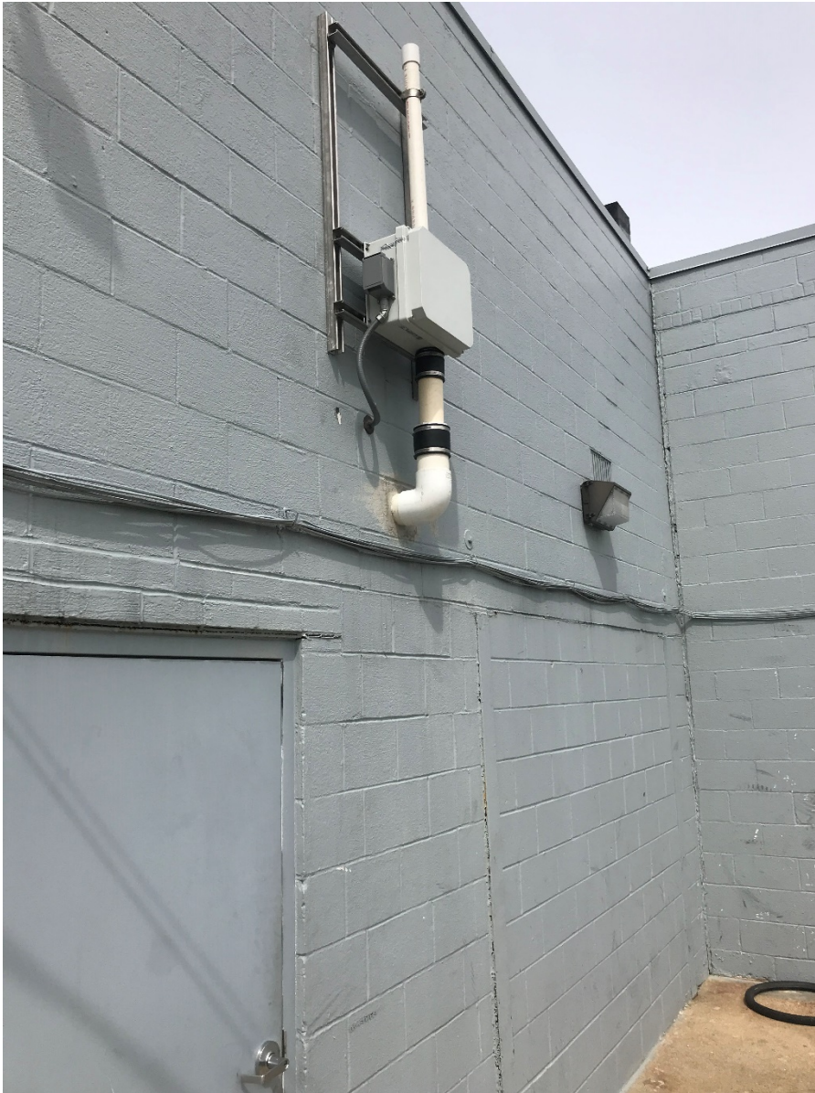
Photo 3: Looking northeast at RadonAway HS200 blower (5/4/20).
