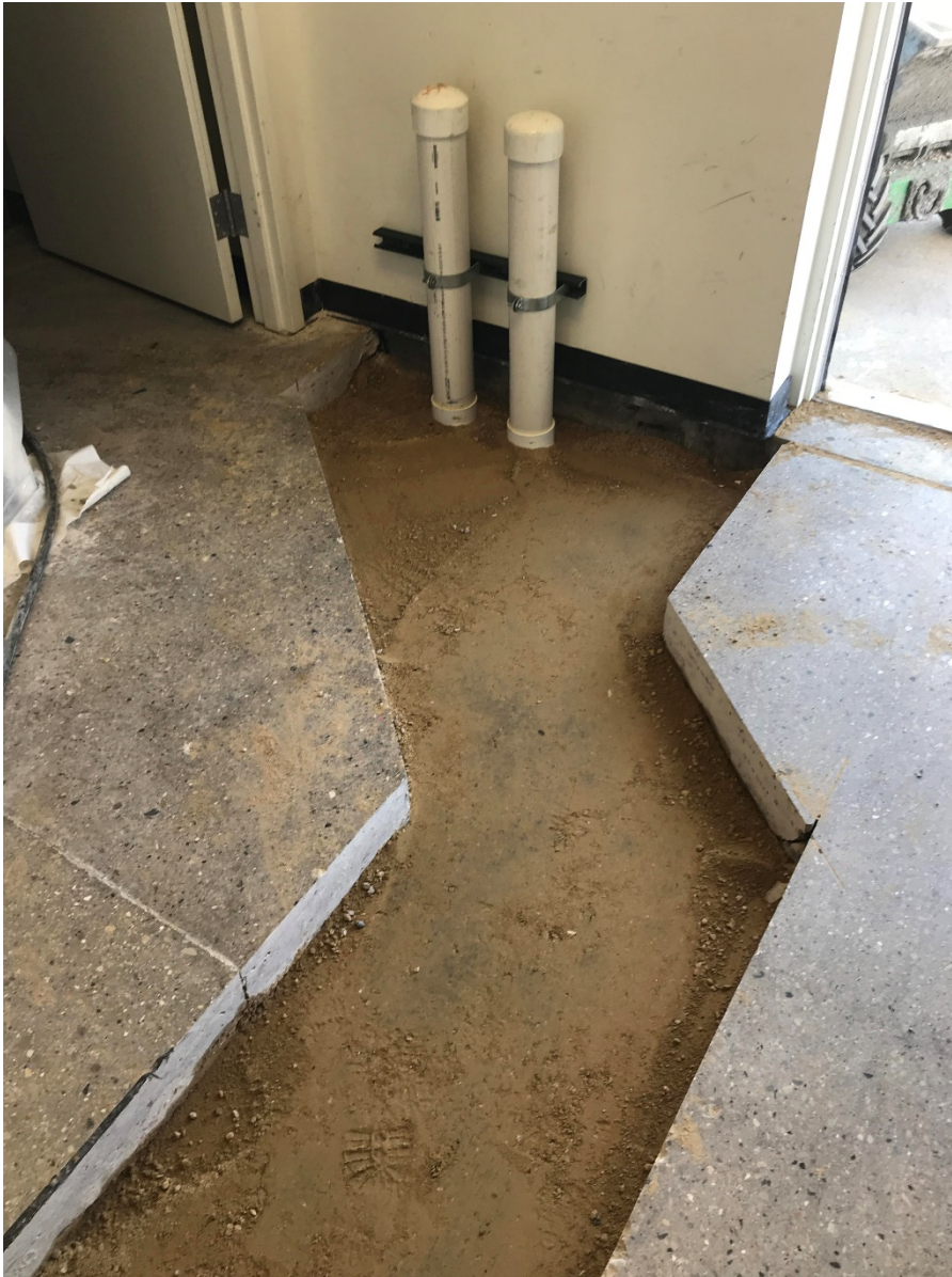
Photo 11: Looking south at vapor mitigation system pipe sub-up and fine-grained soil backfill (3/17/20).
