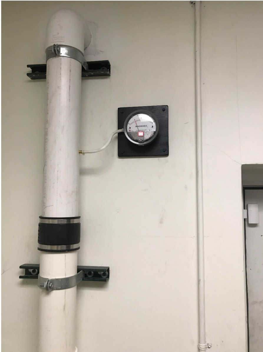
Photo 19: Looking south at vapor mitigation system piping and manometer (5/4/20).
