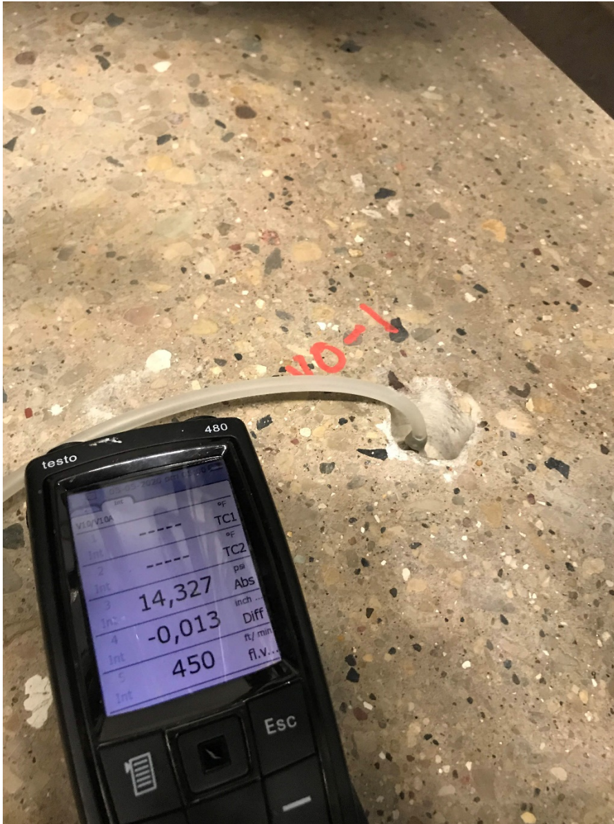
Photo 20: Pressure field extension testing (typical) following system startup (5/5/20).
