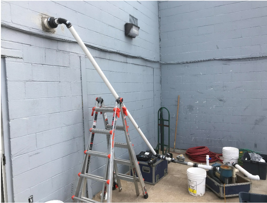
Photo 17: Looking northeast at pilot test equipment (3/24/20).
