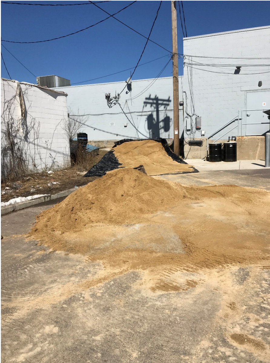
Photo 1: Looking north at south end of Dream Bikes. Limestone screenings ramp constructed to access unit (3/13/20).
