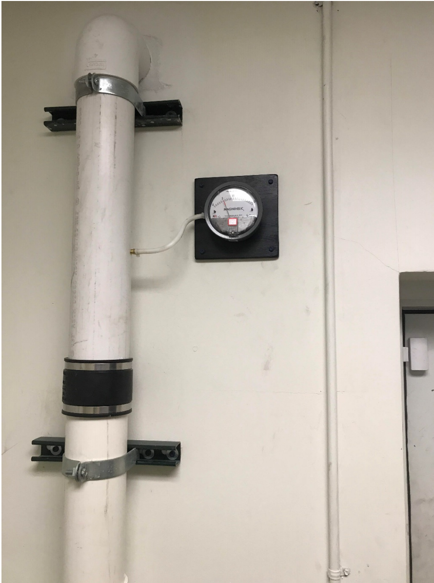
Photo 4: Looking south at vapor mitigation system piping and manometer (5/4/20).
