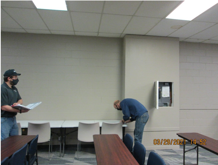
Photo 3: Pick-up point 30 location adjacent build out. Electrical panel shown. This is H&R Block training area in back of the client area.
