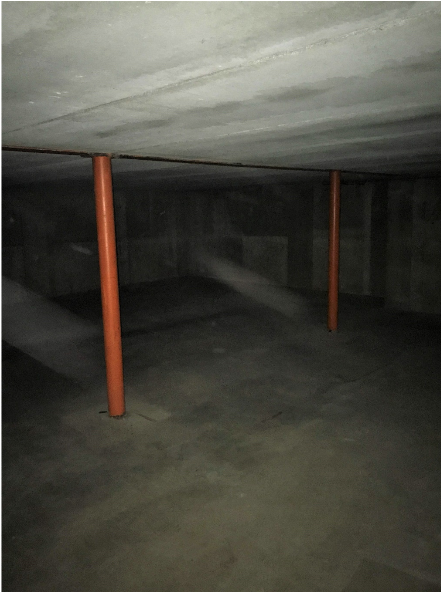
Photo 7: Abandoned basement – Dream Bikes side access.
