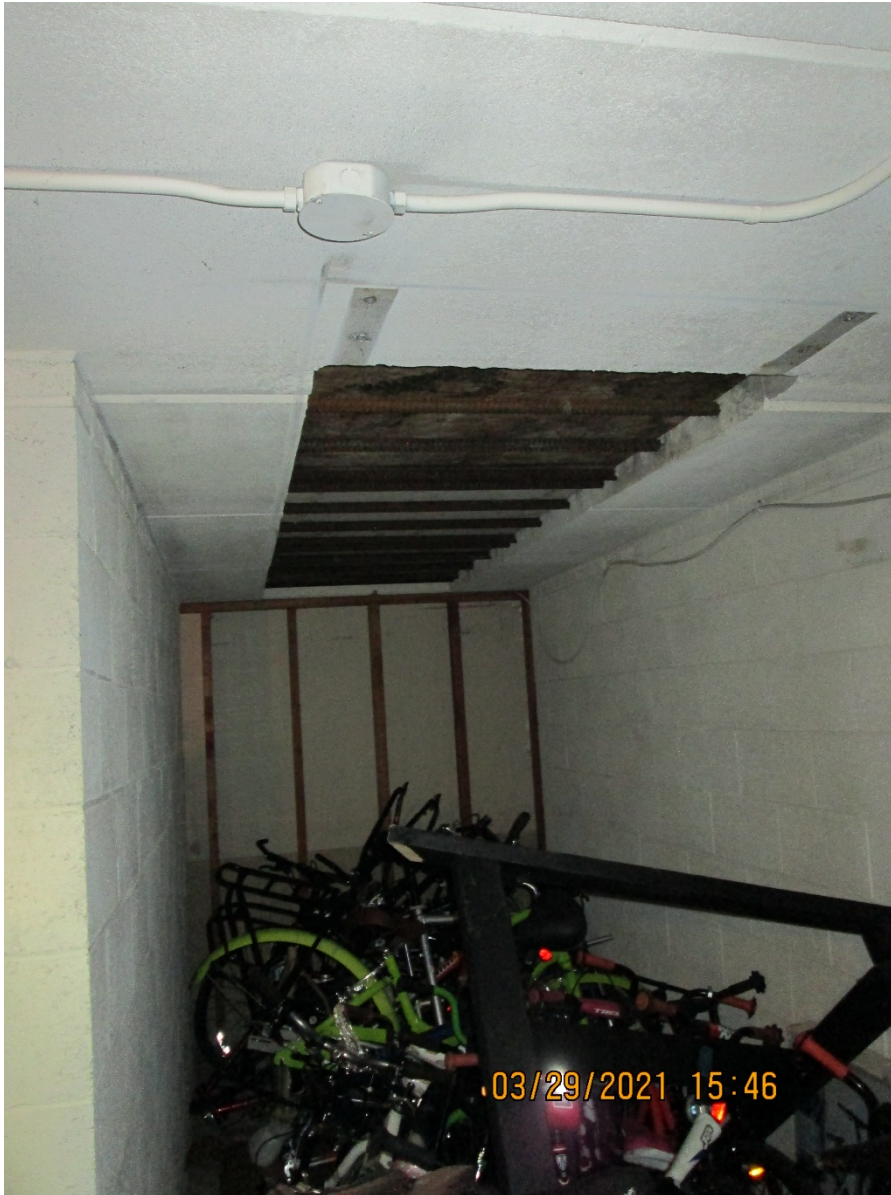
Photo 5: Unit 1117 basement ceiling.
