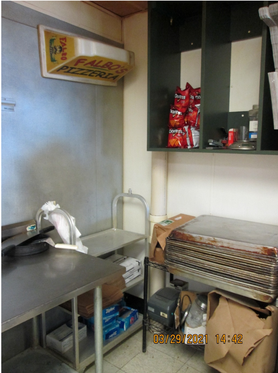
Photo 5: Possible location for pick-up point 31 near corner along walk-in-cooler. Vertical pipe shown is a roof drain connected to the storm sewer. The wall between Falbos and H&R Block is a build out (not an original wall).
