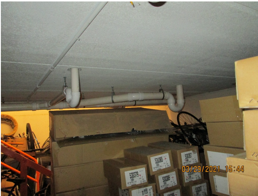
Photo 4: Unit 1117 basement ceiling.
