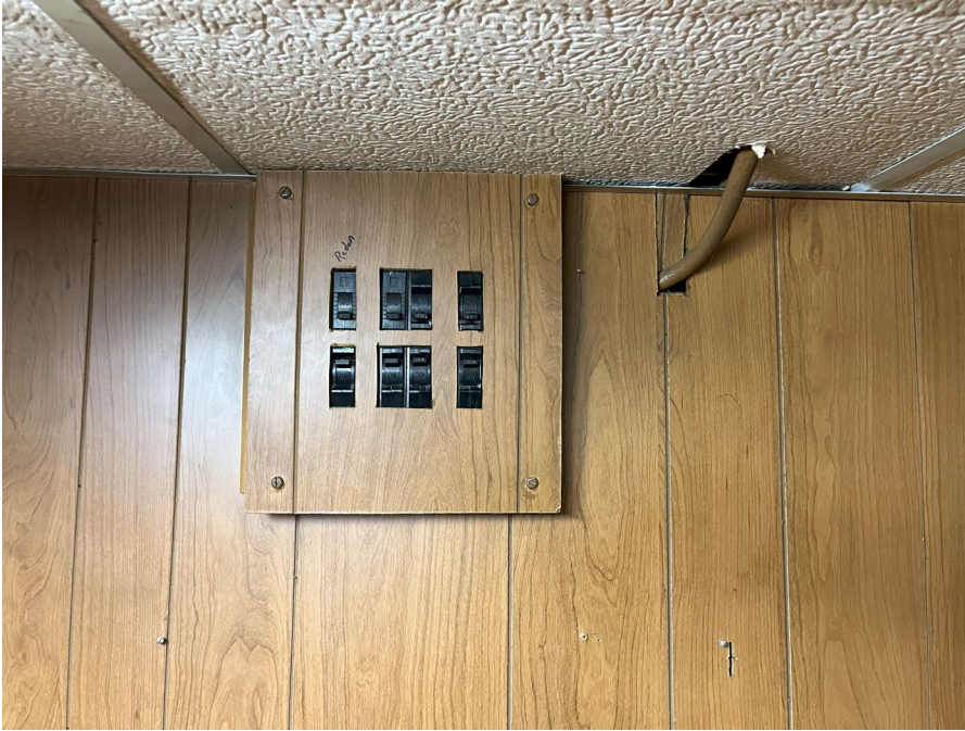
Photo 7: Looking north at breaker panel inside office at northwest corner of basement. Breaker at upper left is labeled "Radon" for radon/mitigation fan.
