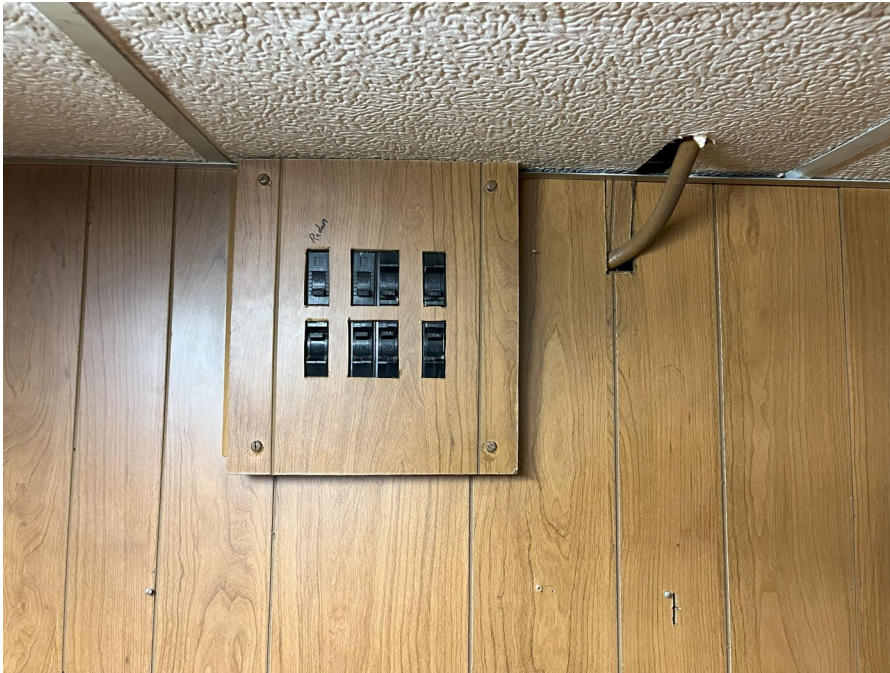
Photo 7: Looking north at breaker panel inside office at northwest corner of basement. Breaker at upper left is labeled "Radon" for radon/mitigation fan.
