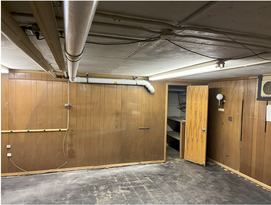
Photo 5: Looking east at piping which comes from the moisture drop line inside the closet and runs to Pickup #2.
