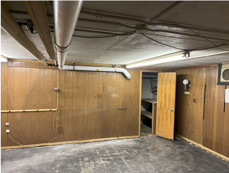
Photo 5: Looking east at piping which comes from the moisture drop line inside the closet and runs to Pickup #2.
