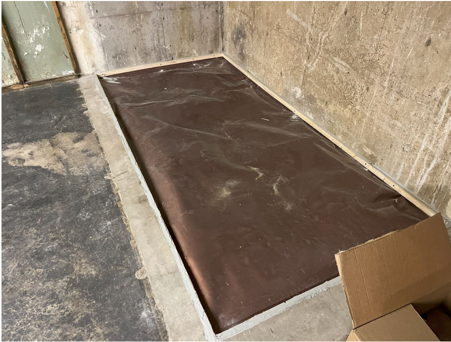
Photo 11: Looking southwest at Dregro Wrap vapor barrier covering opening in floor where fuel oil tank sat.
