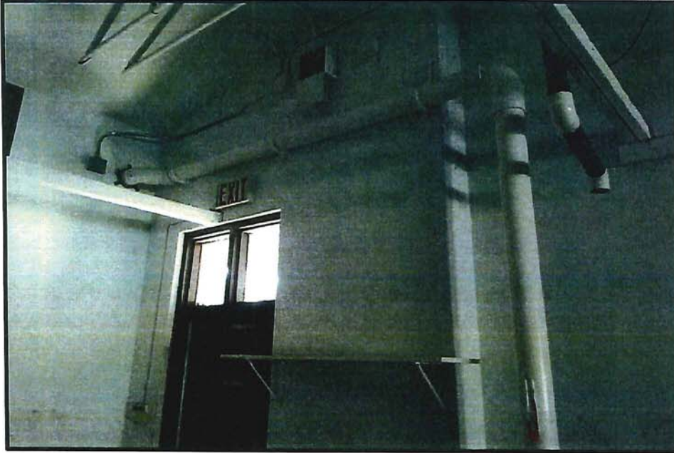
Photo 5 – This photograph shows the upper PVC piping of the VMS and the exit point through the wall. This photograph also shows that the exterior fan is hardwired to the internal power source.
