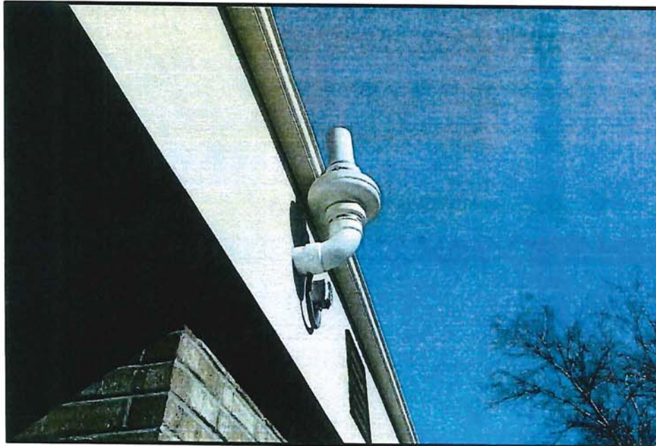
Photo 7 – This photograph looks northeast and up at the exterior fan
