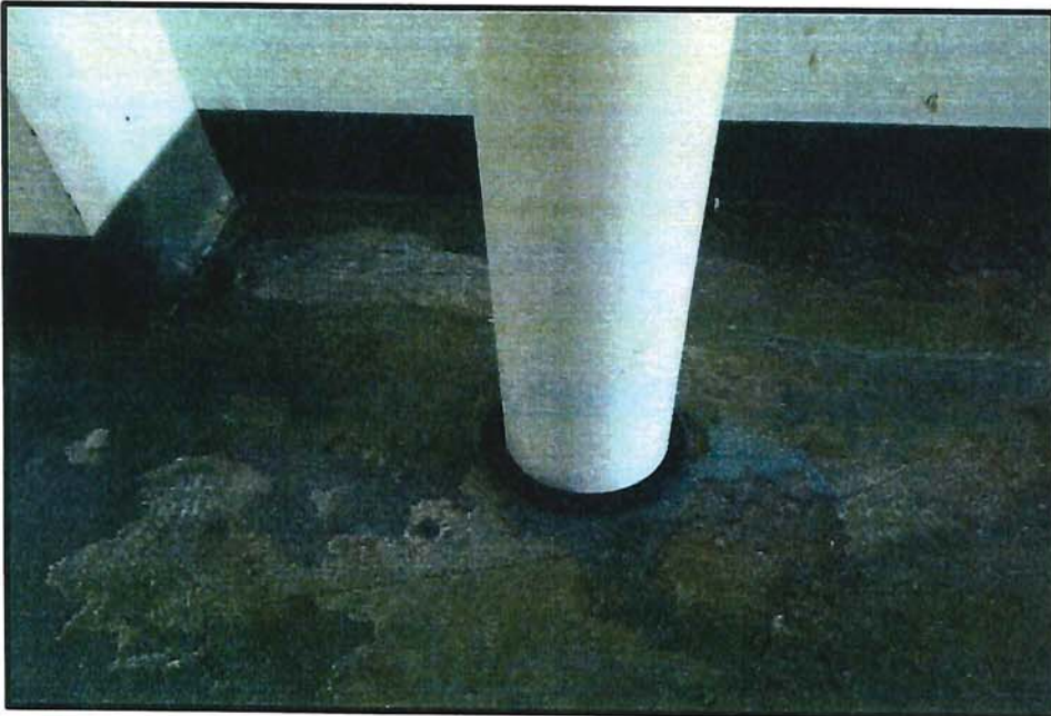
Photo 3 – This photograph shows a close up of the floor penetration of the VMS. The floor penetration was sealed with a rubber gasket and caulk. The concrete is approximately 5 to 6 inches thick and approximately 5 inches of sub slab concrete was removed.
