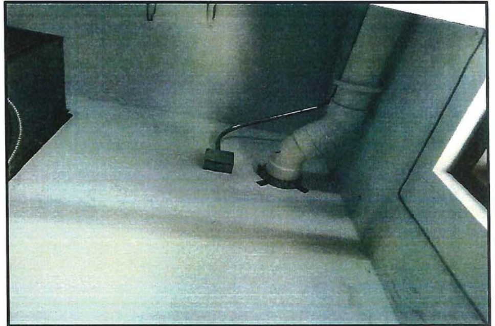
Photo 6 – This photograph shows a close up of the exit point and the interior electrical junction box.
