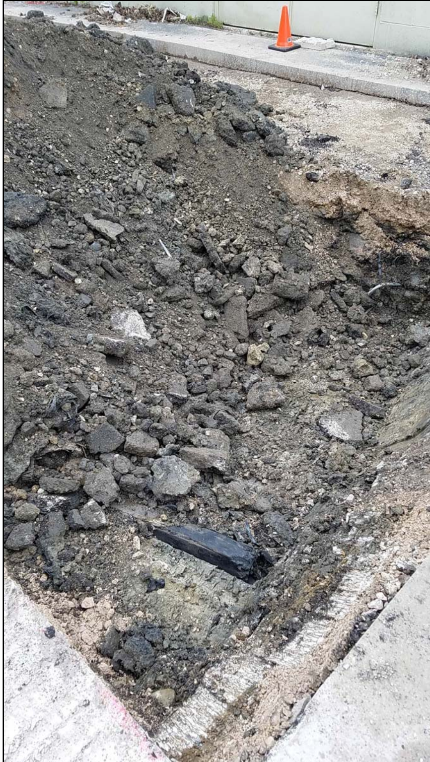
Debris in fill material
