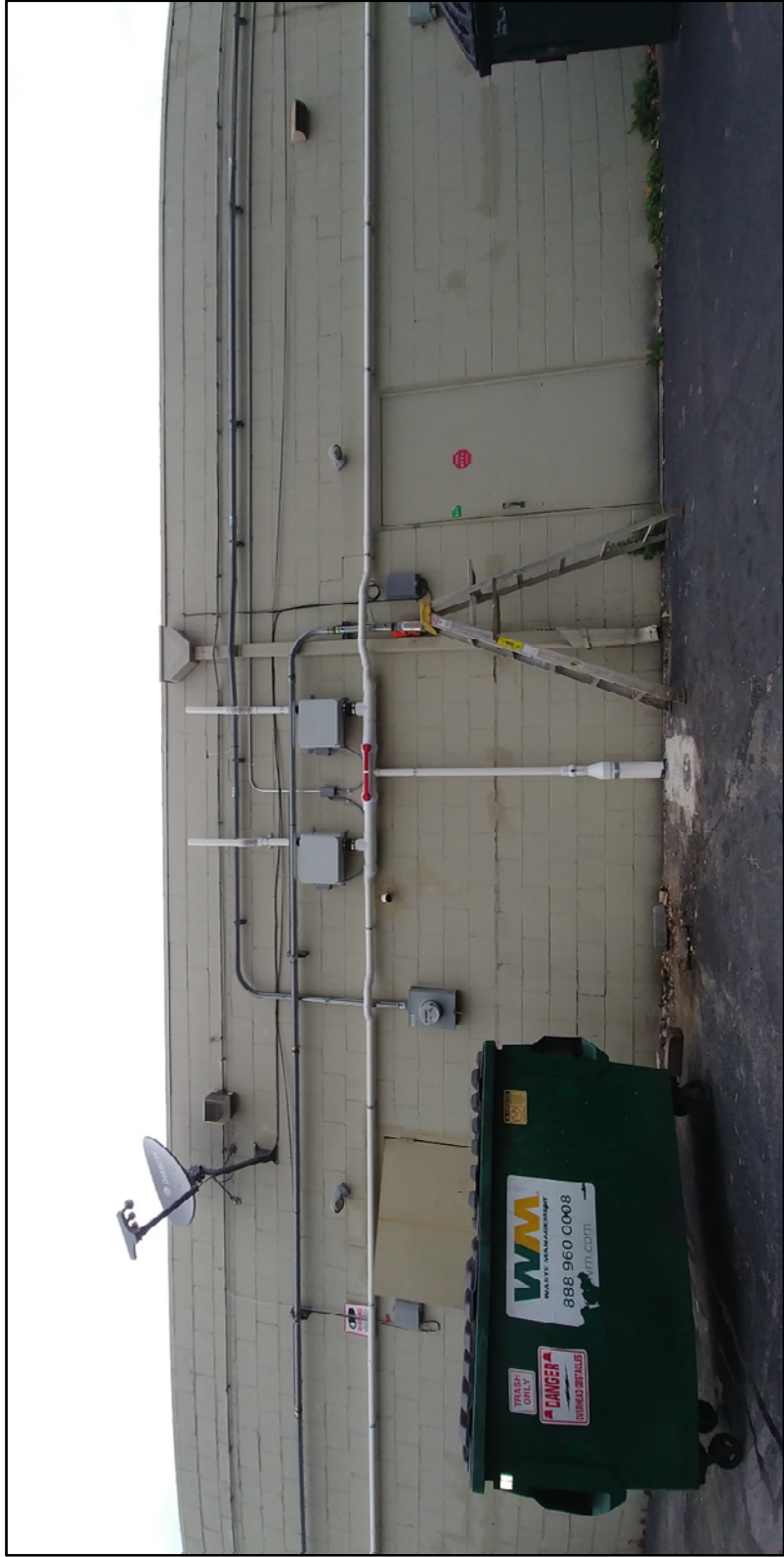
Overview of the SVE system. Extraction well SVE-2 and the fans are shown in the photo.
