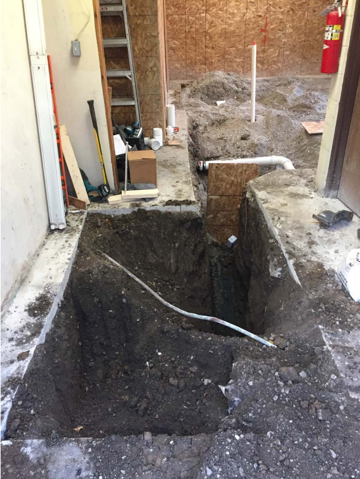
Photo 3, November 22, 2016. Overview of interior excavation area, facing north. The door shown on the right edge of the photo leads into the mechanical equipment room containing a boiler, compressor, water heater, etc. The room is surrounded by a concrete block wall that comprised a structural impediment to expanded excavation inside the building.
