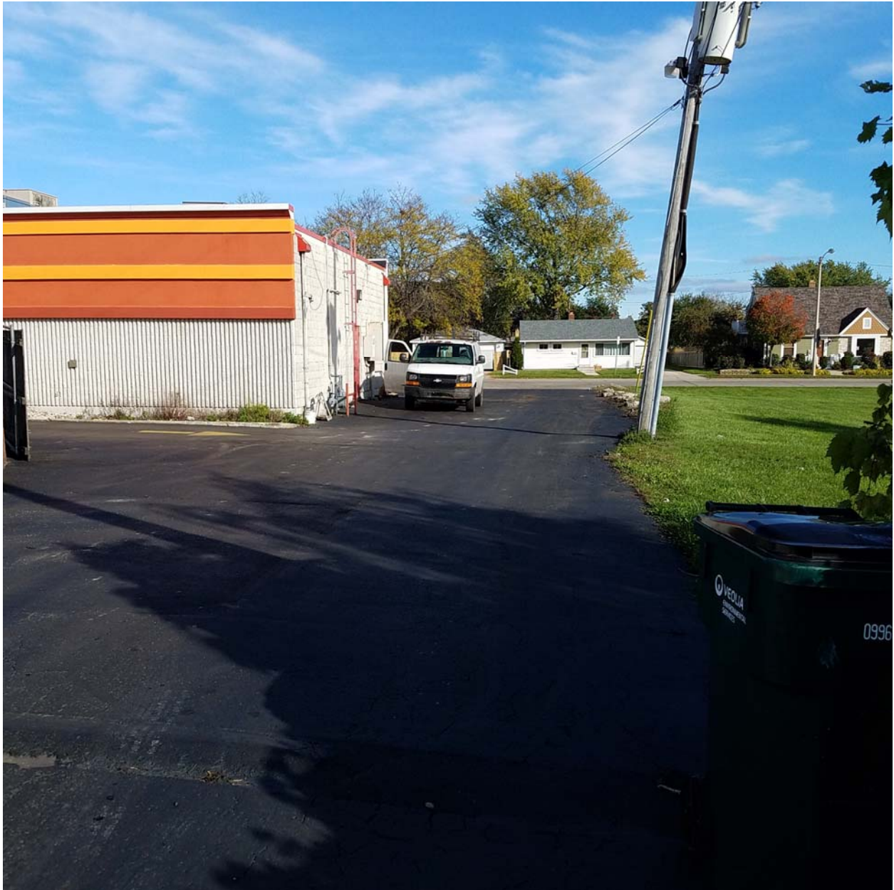
Overview of alleyway portion of the asphalt cap south of 3909 52 nd Street, facing east
