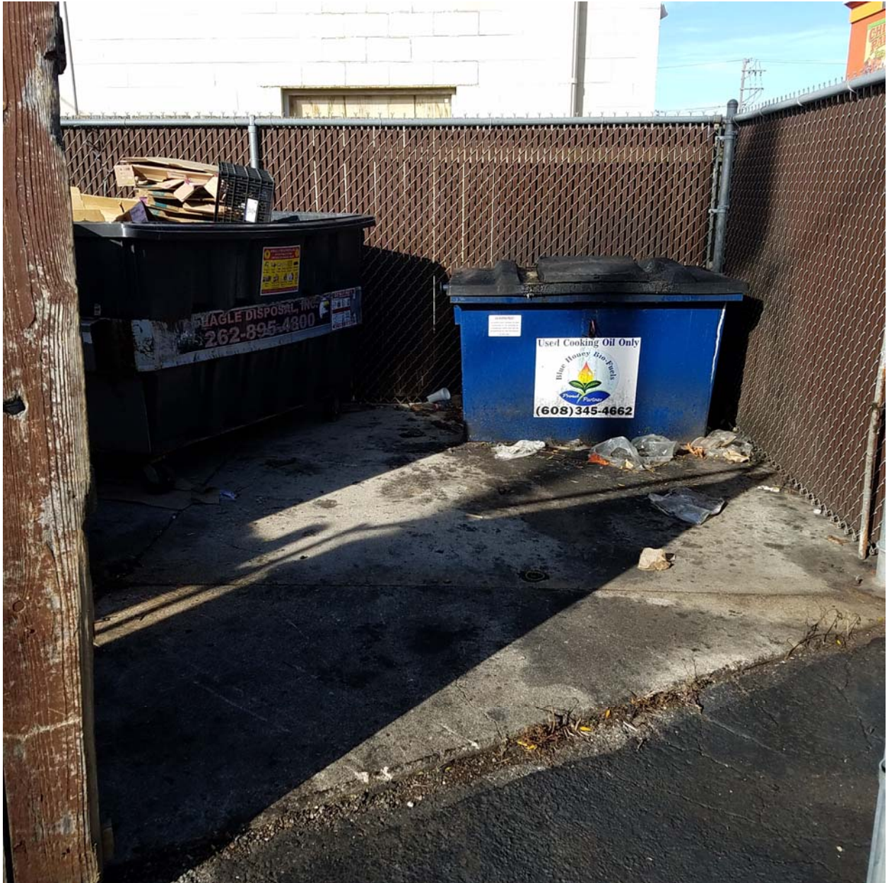
Concrete cap in trash corral south of 3909 52 nd Street
