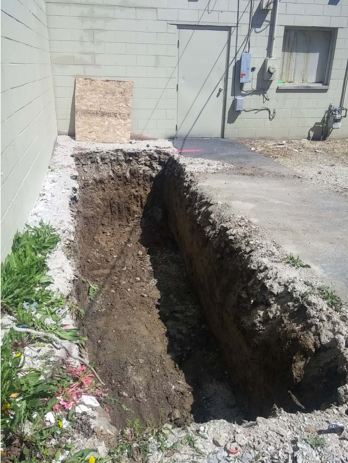
Photo 1, May 10, 2017. Overview of exterior excavation area 2, facing north. The exterior building walls (and footings) were structural impediments to expanded excavation west toward the source area.
