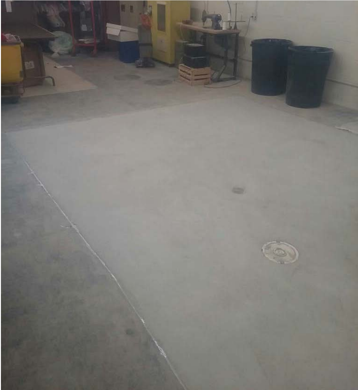
Concrete cap (building floor slab) inside 3917 52 nd Street, including excavation repair and seal.
