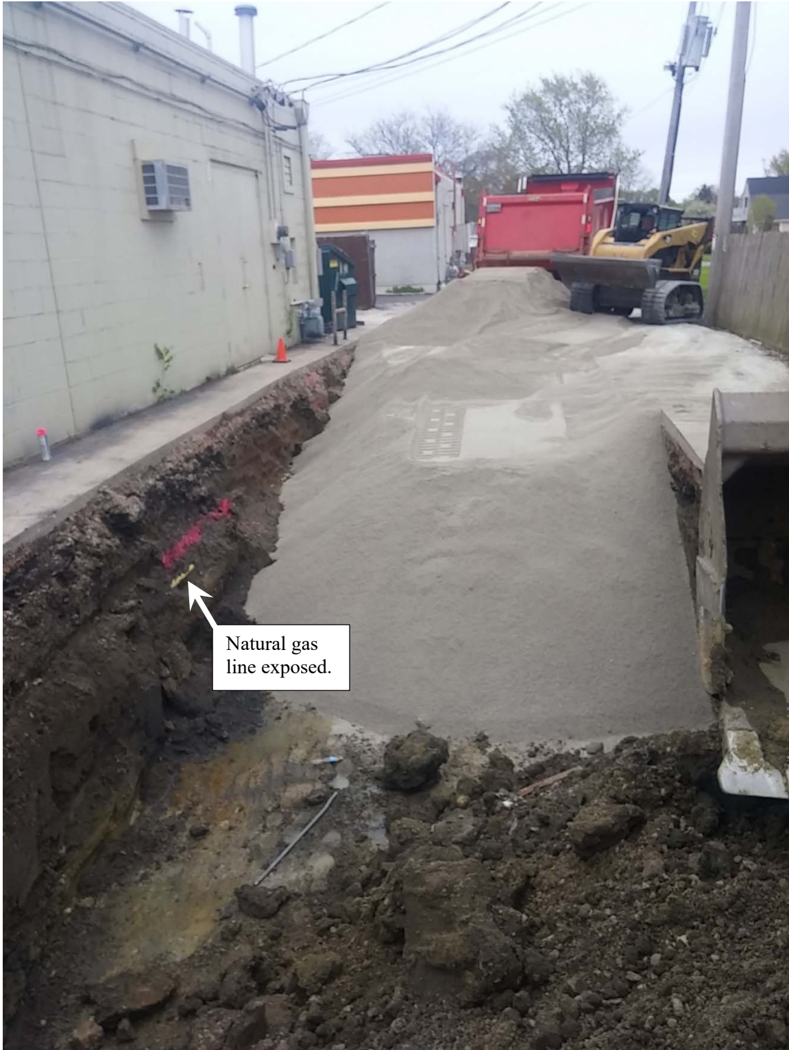
Photo 2, May 9, 2017. Overview of exterior excavation area 1, facing east. The exterior building wall (and footing), and utility lines along the wall, were structural impediments to expanded excavation toward the source area.
