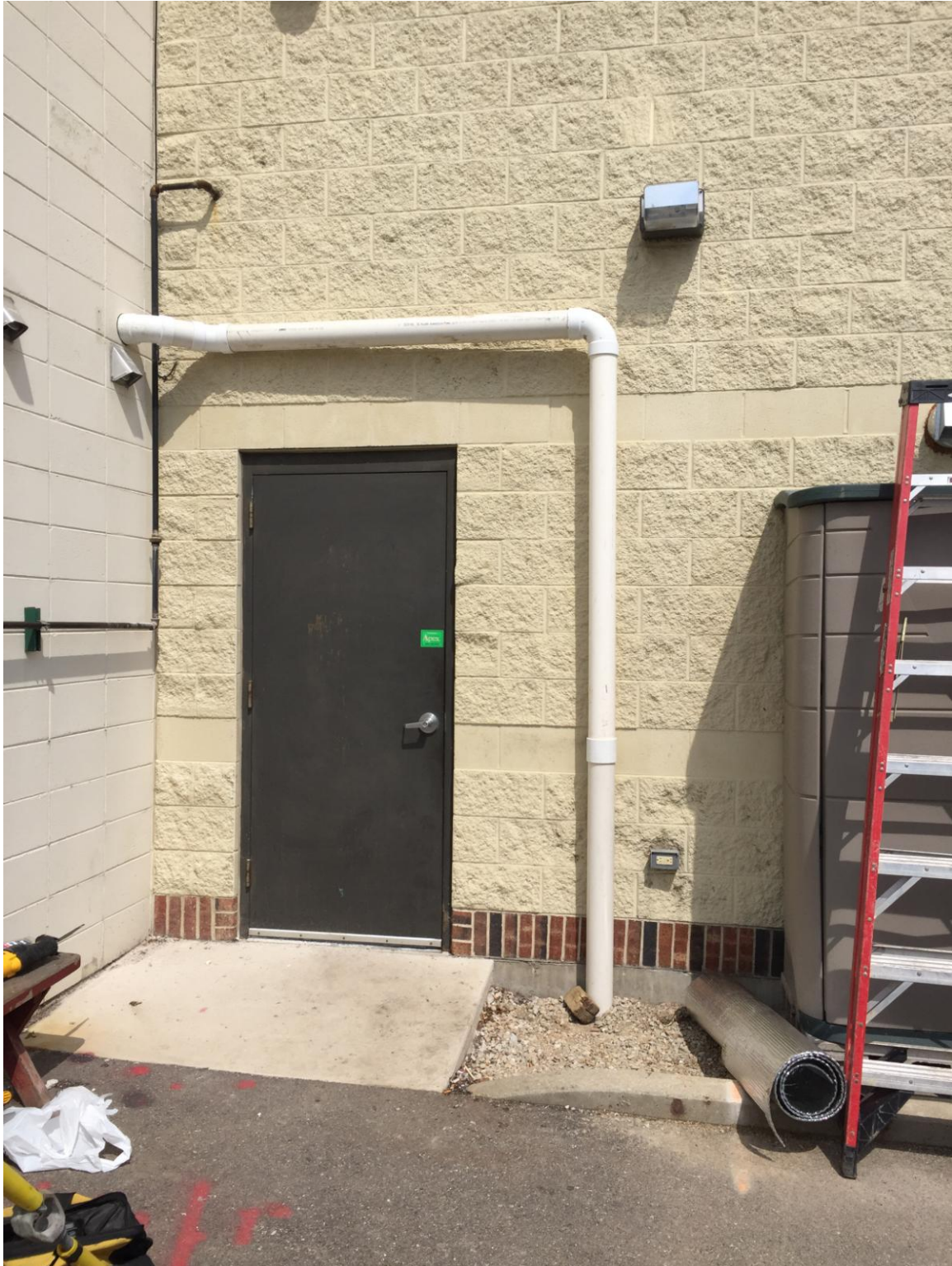
Conveyance line coming from SVE-2 to the trenched section on the south side of the building.
