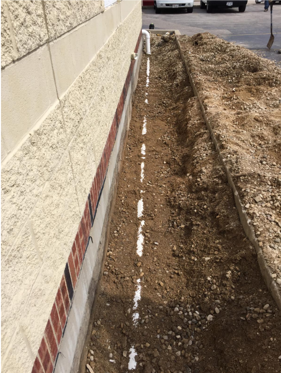
Conveyance piping set to 2 feet bgs. Soil added in trench and leveled off for the addition of R-board installation over the top of the PVC.
