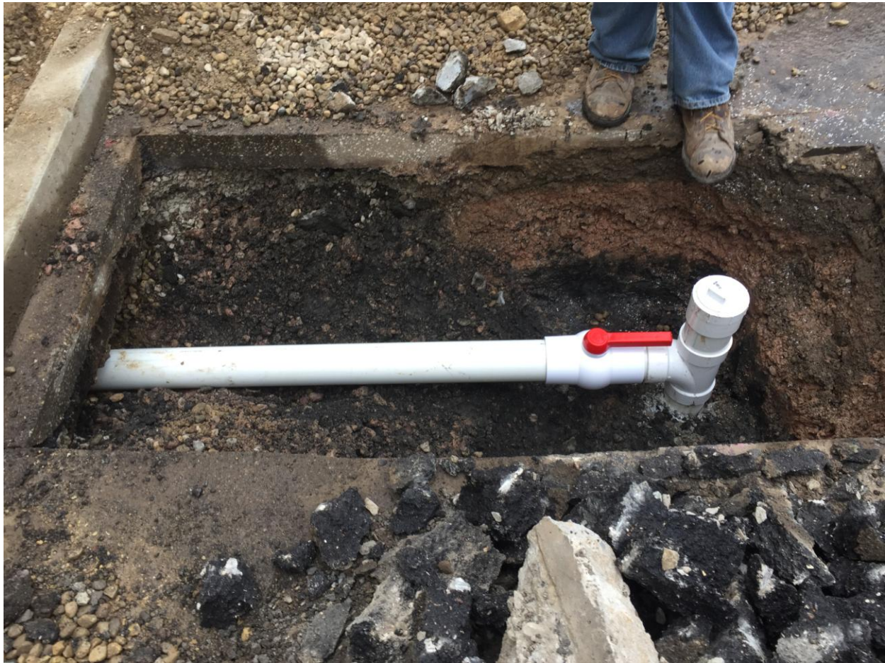
Ball valve and clean-out added to SVE-1, and pipe connecting the well to the main conveyance line.
