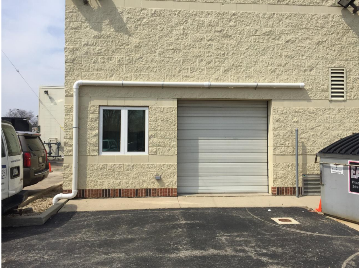
Above ground conveyance line installed on the east side of the building.
