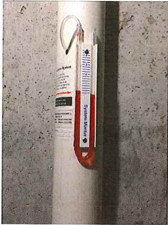
Photo #1 U-Tube Liquid Manometer Located In Building Basement
