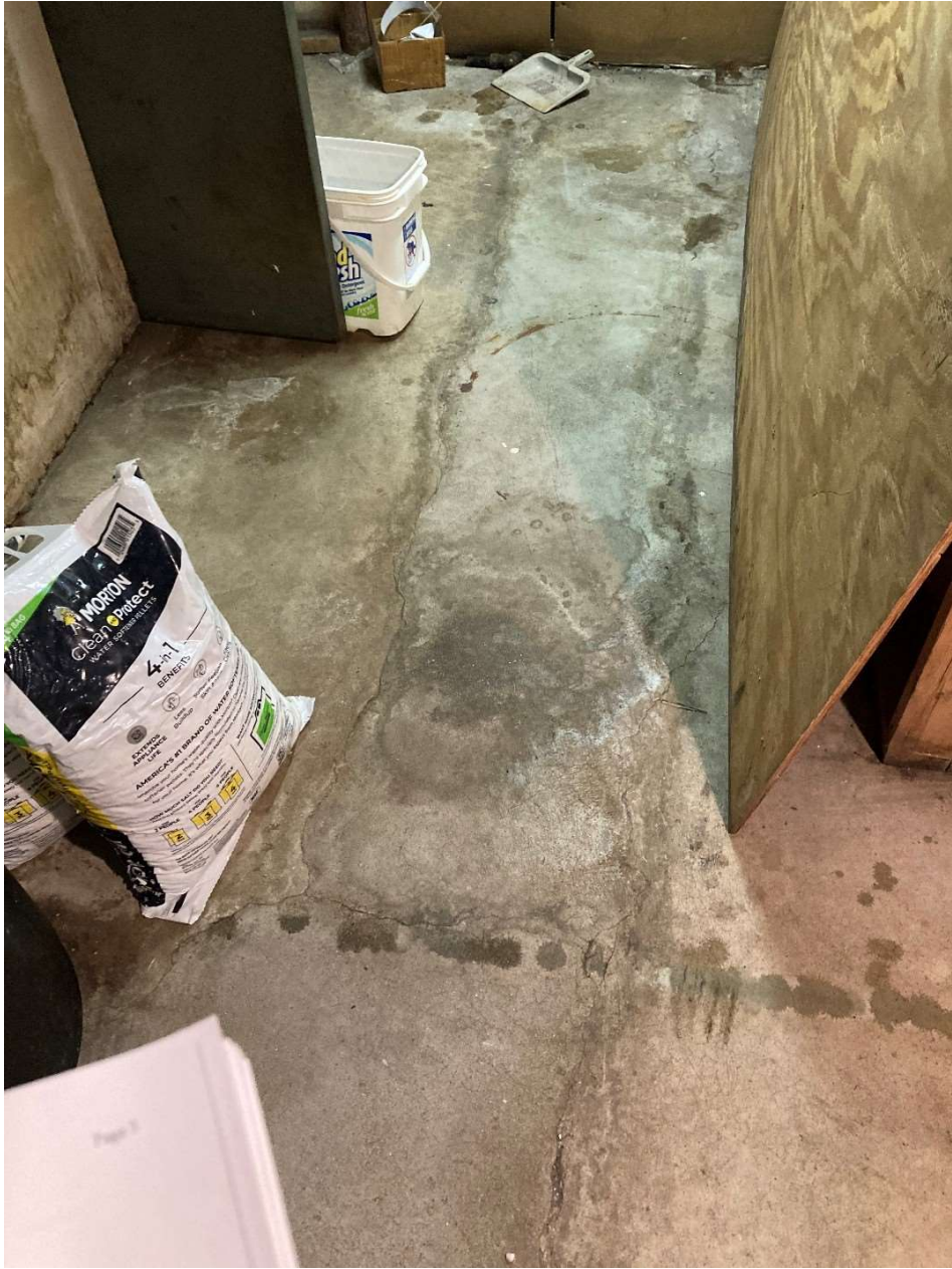
Basement Floor – Slight cracking
