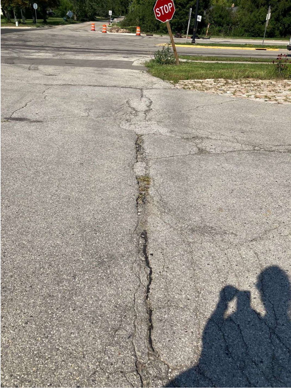
Entrance to property off N. Port Washington Road – Crack in asphalt pavement
