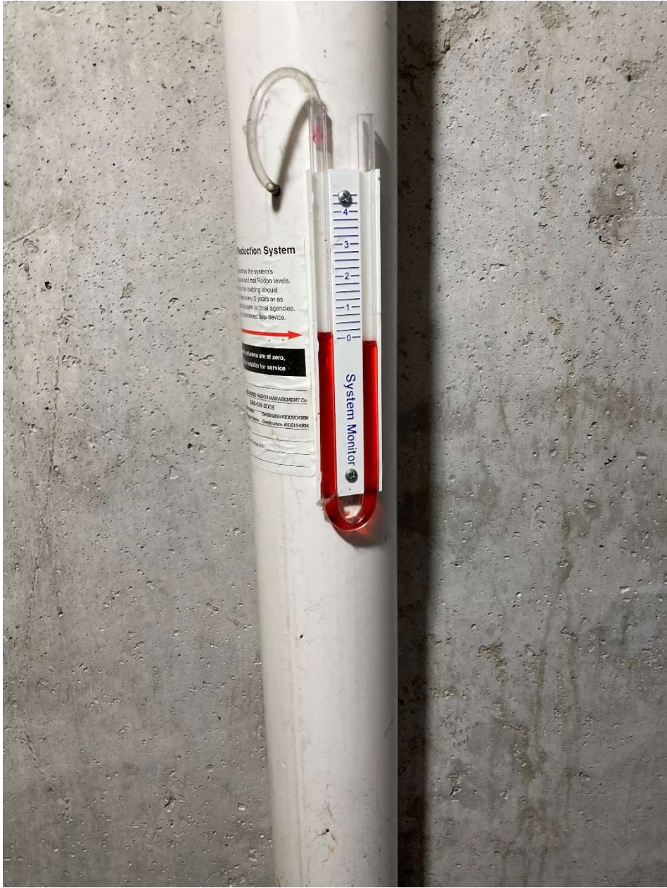
U-Tube Liquid Manometer located in building basement
